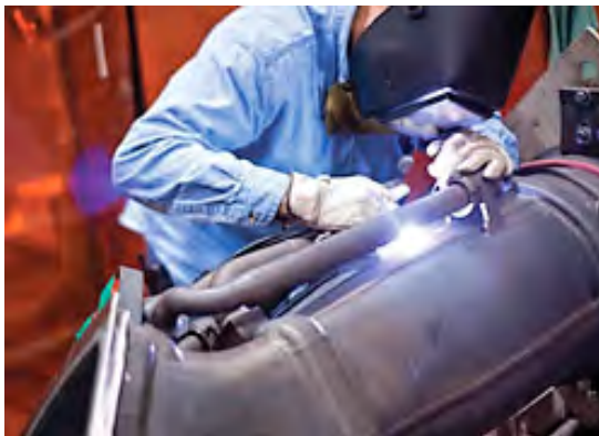
Photo- 9: Welding of GT combustor (MHI)
