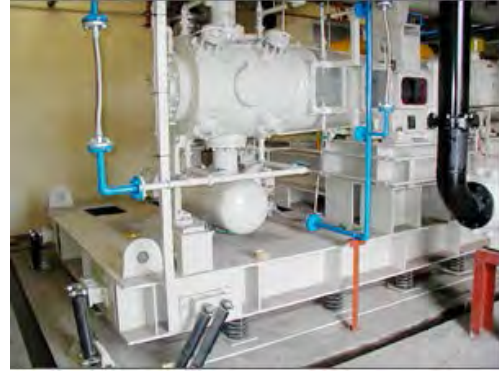
Photo- 3: Isolated base for compressor
