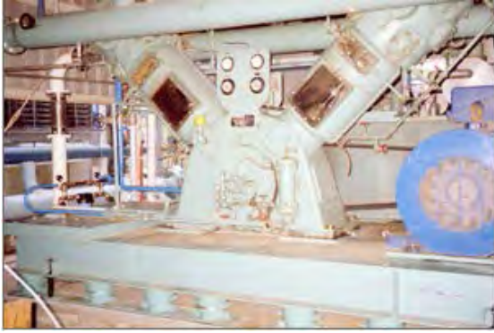
Photo- 2: Isolated base for compressor
