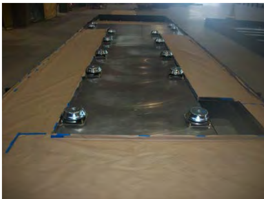
Photo- 5: Vibration isolator for gen. set
