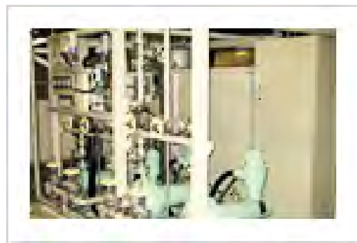
Photo- 6: Oxygen gas injection equipment
