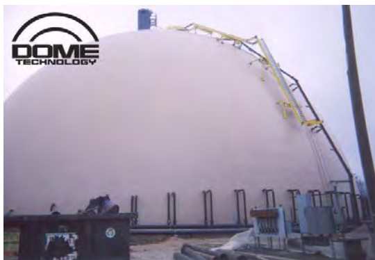
Photo- 23: Fly-ash silo
