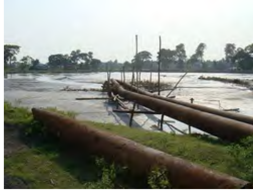
Photo- 15: Coal ash slurry pipe
