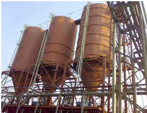
Photo- 21: Fly-ash silo
