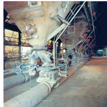
Photo- 10: Air slide conveyor
