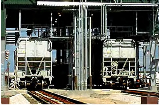
Photo- 27: Fly-ash loading facility
