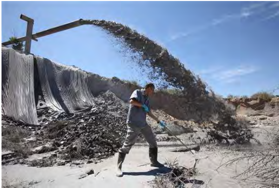
Photo- 41: Low Density Slurry Discharge
