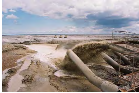
Photo- 42: Low Density Slurry Discharge
