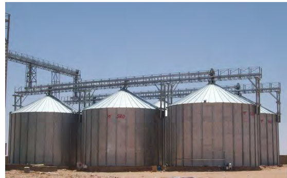
Photo- 22: Fly-ash silo
