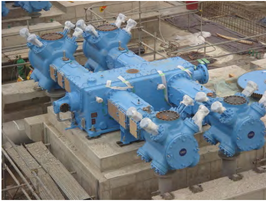
Photo- 44: BCG compressor
