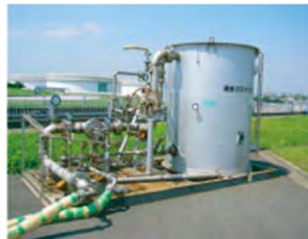
Photo- 43: Hot bath N 2 vaporizer
