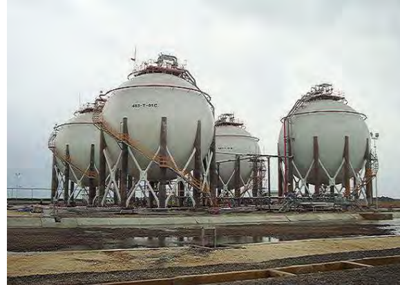
Photo- 31: LPG tank
