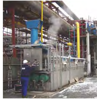
Photo- 48: Submerged combustion vaporizer
