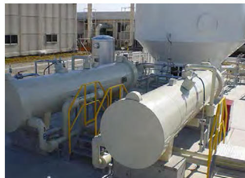
Photo- 50: Hot water type vaporizer
