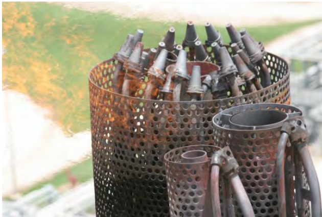
Photo- 51: Flaire stack pilot burner
