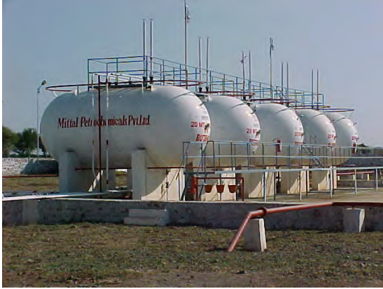
Photo- 30: LPG tank
