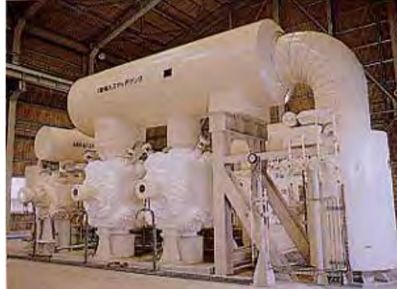
Photo- 45: BCG compressor
