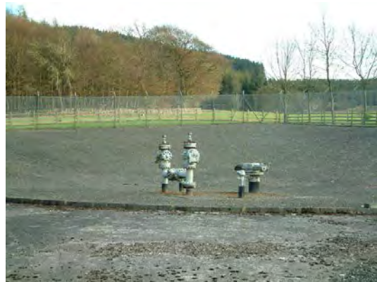
Photo- 18: Venting station on natural gas pipeline
