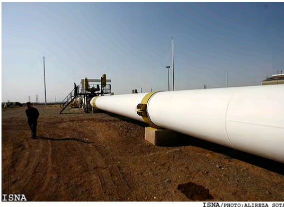
Photo- 19: Natural gas pipeline on land
