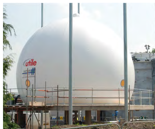
Photo- 49: Membrane gas holder
