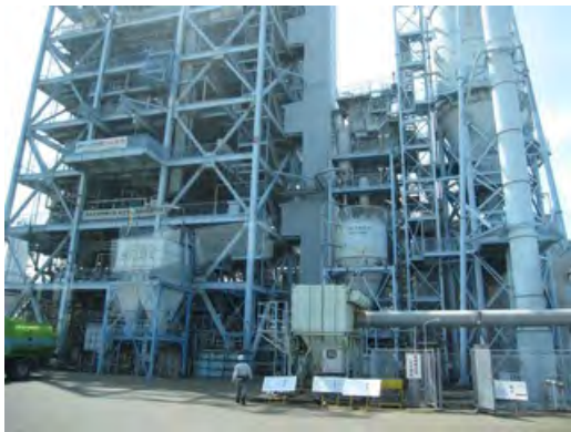
Photo- 40: Gas generation plant
