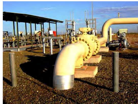
Photo- 20: Natural gas pipeline on land
