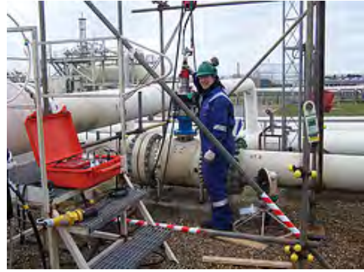
Photo- 14: Flange joint
