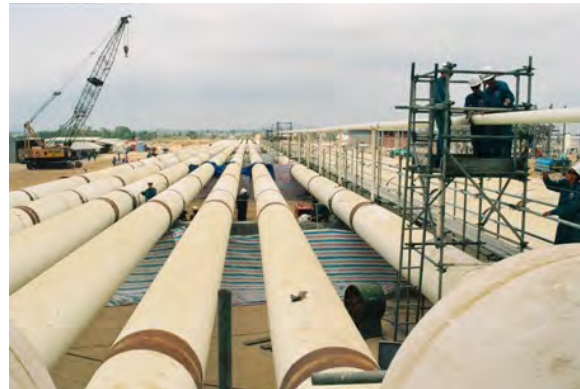
Photo- 5: Natural gas pipeline in Nam Con Son
