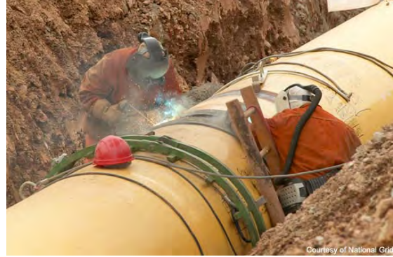
Photo- 11: Buried gas pipeline
