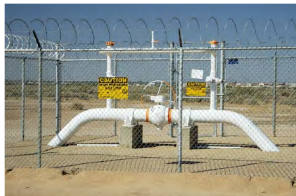
Photo- 22: Shutoff valve for Natural gas pipeline
