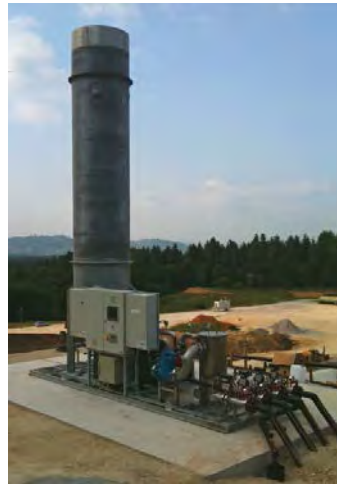
Photo- 43: Landfill gas flaire stack
