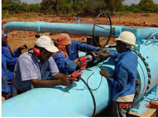
Photo- 13: Flange joint
