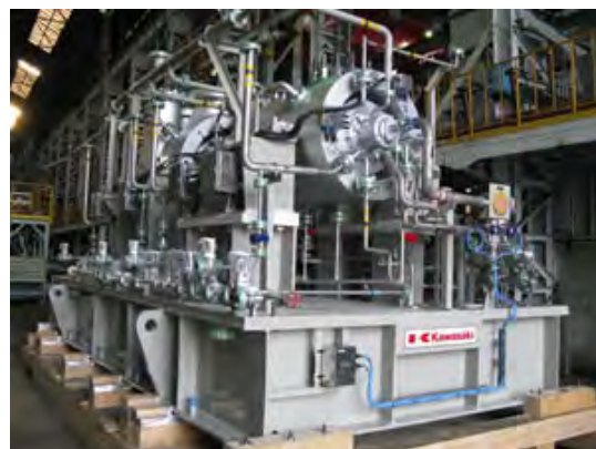
Photo- 2: Gas compression module
