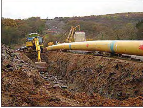
Photo- 10: Buried gas pipeline
