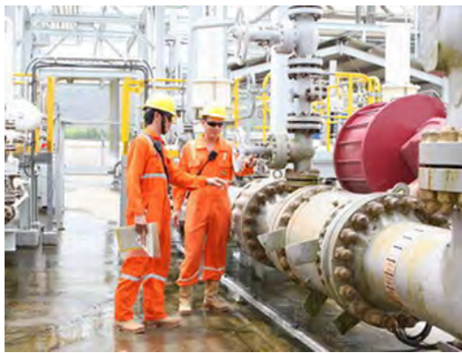
Photo- 6: Natural gas pipeline in Nam Con Son
