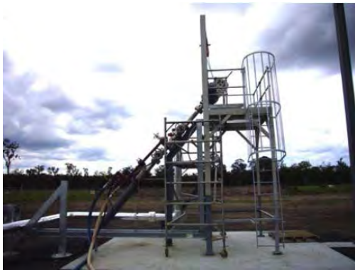
Photo- 39: Production well (Carbon energy)
