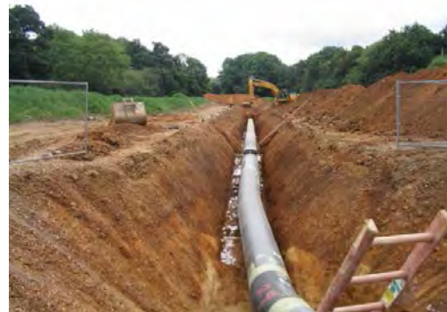
Photo- 9: Buried gas pipeline
