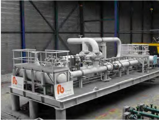
Photo- 22: Ultrasonic fiscal metering skid
