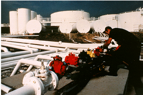
Photo- 119: Oil receiving pipe
