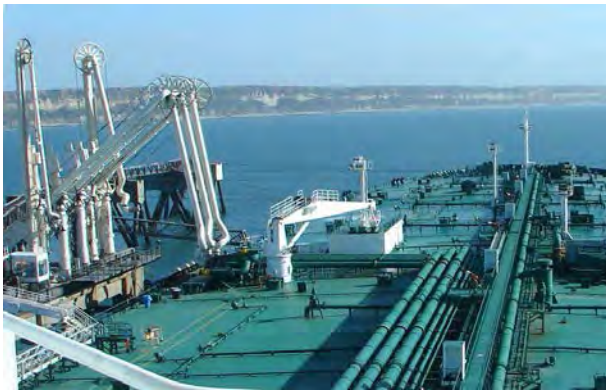
Photo- 5: Oil unloading facility
