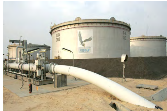
Photo- 25: Crude oil receiving metering facility
