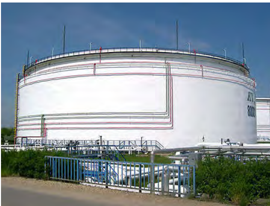
Photo- 109: Crude oil tank
