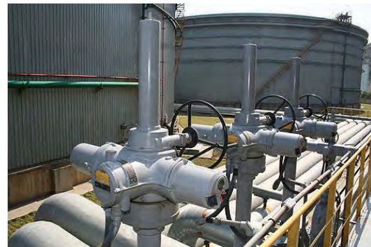
Photo- 118: Switching ball valve
