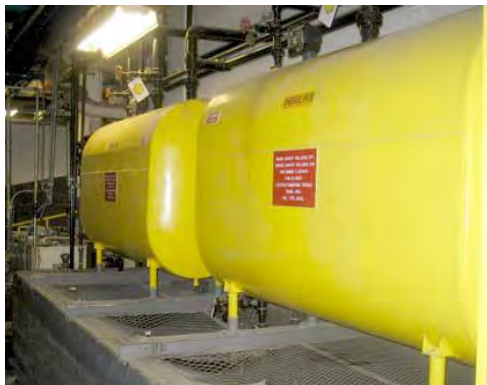
Photo- 114: Indoor oil storage tank
