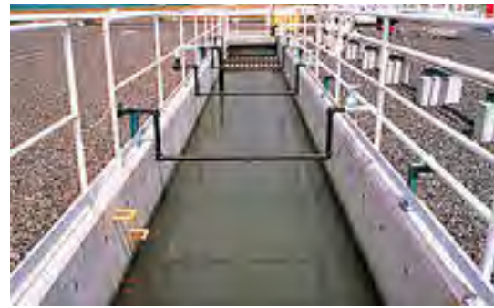
Photo- 130: API oil separator
