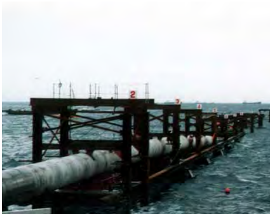
Photo- 69: Offshore pipeline for crude oil
