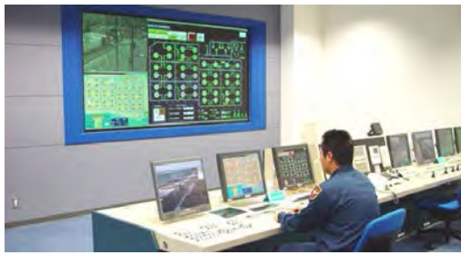
Photo- 88: Central monitoring board
