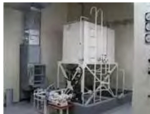
Photo- 115: Fuel dispensing tank
