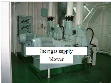
Photo- 15: Inert gas supply blower
