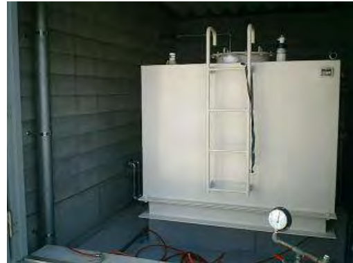
Photo- 113: Indoor oil storage tank
