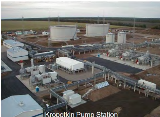
Photo- 24: Pumping station
