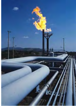
Photo- 42: Expansion bend of pipeline
