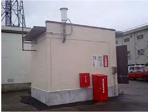
Photo- 112: Indoor oil storage house
