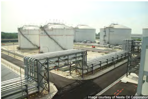
Photo- 116: Piping around oil tank
