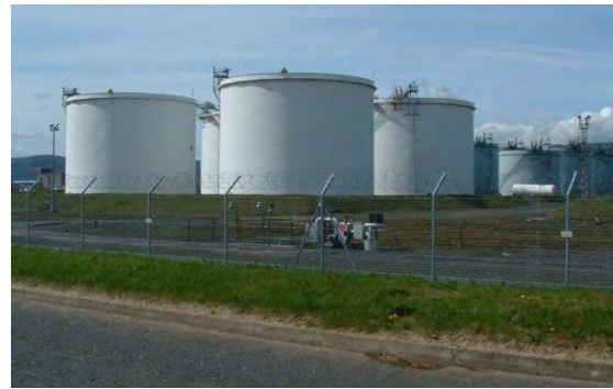
Photo- 104: Outdoor oil storage tank
