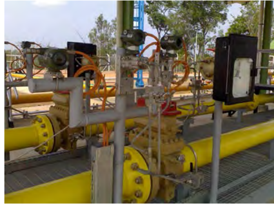
Photo- 23: Metering system
