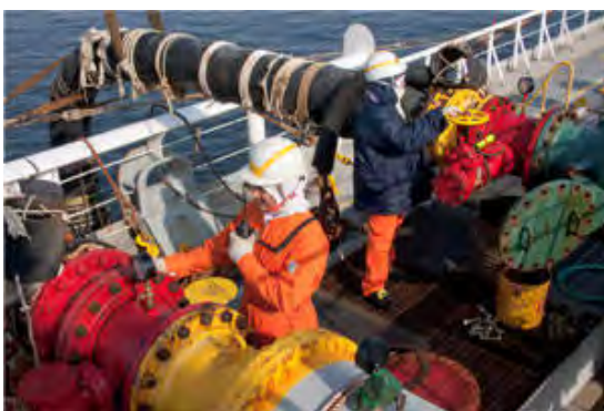
Photo- 17: Marine hose for unloading
