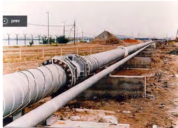
Photo- 59: Trace heater for heavy oil
