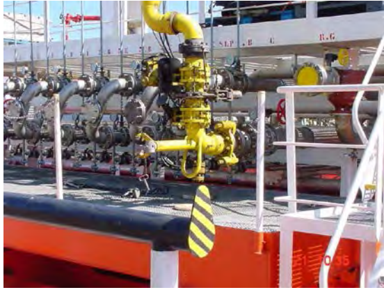
Photo- 9: Oil unloading coupler
