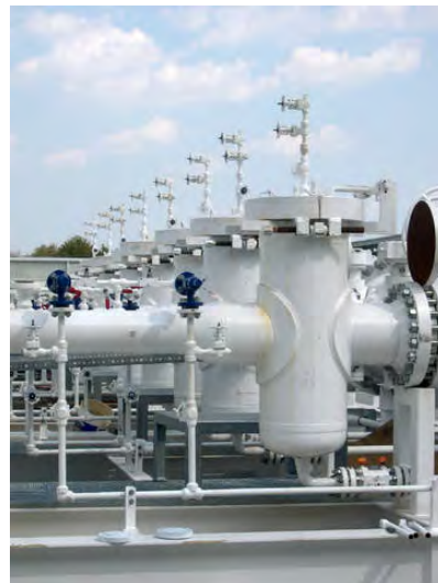
Photo- 21: Line strainer
