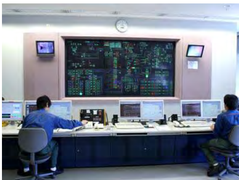
Photo- 27: Control room for oil pipeline
