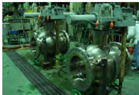
Photo- 30: Shut-off valve between marine hose and subsea pipeline
