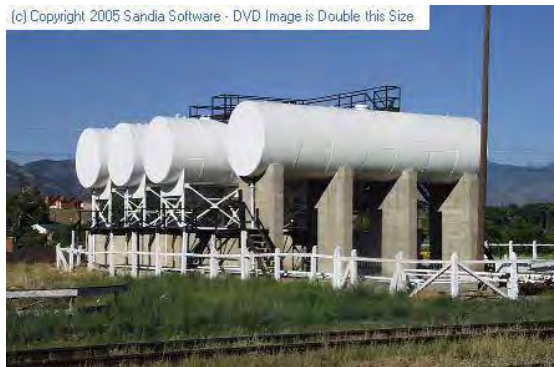
Photo- 105: Outdoor oil storage tank
