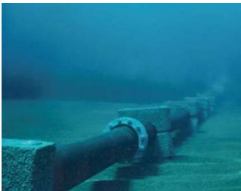
Photo- 70: Pipeline on the seabed
