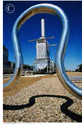
Photo- 43: Expansion bend of pipeline
