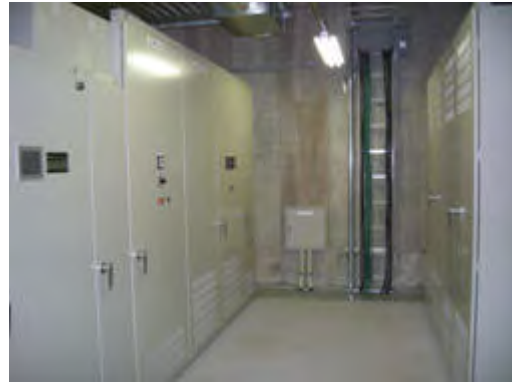
Photo- 101: Uninterruptible power supply
