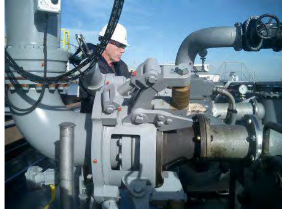
Photo- 10: Oil unloading coupler
