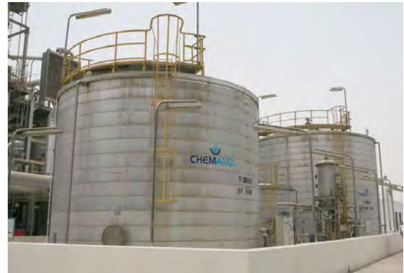
Photo- 127: Outdoor oil storage tank
