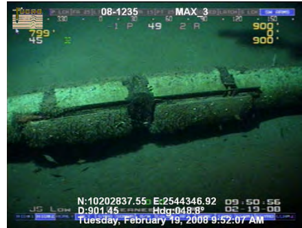
Photo- 53: Deepwater cathodic protection
