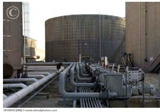
Photo- 117: Piping around oil tank
