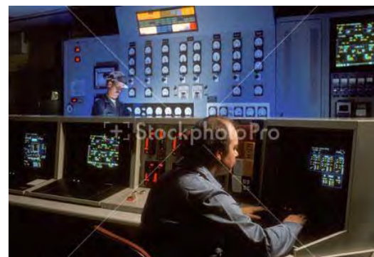
Photo- 28: Control room for oil pipeline
