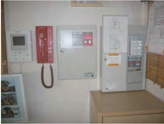
Photo- 39: Fire reporting system
