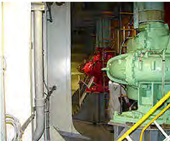
Photo- 41: Crago pump of VLCC
