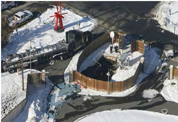
Photo- 94: Underground valve pit
