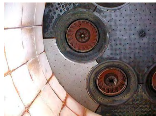
Photo- 12: HBR combustion chamber for V94.2
