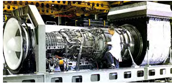
Photo- 4: 28MW class GT (GE-LM2500)
