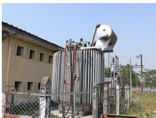
33/6.6kV Transformer in Hluttaw SS
