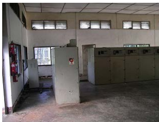
Distribution panel in Hluttaw SS
