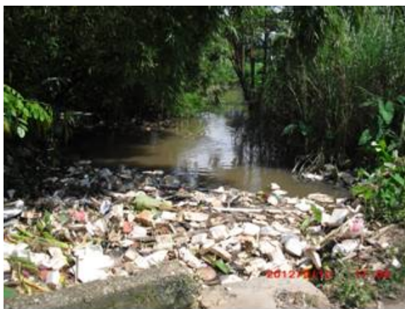
Kathwe Chaung Channel (No.2) No clearance
