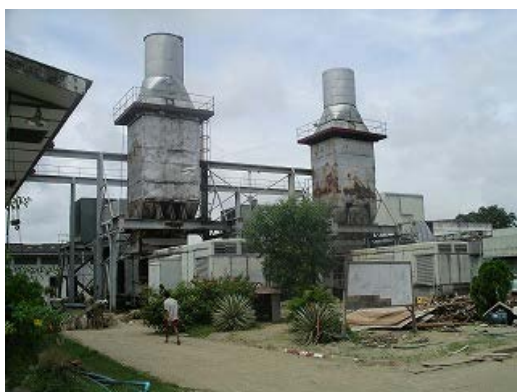
18.45MW Gas turbine power facility in Ywama PS
