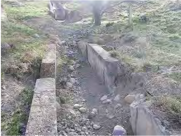
Photo 6-2-56: Damaged Spillway from Head Tank
