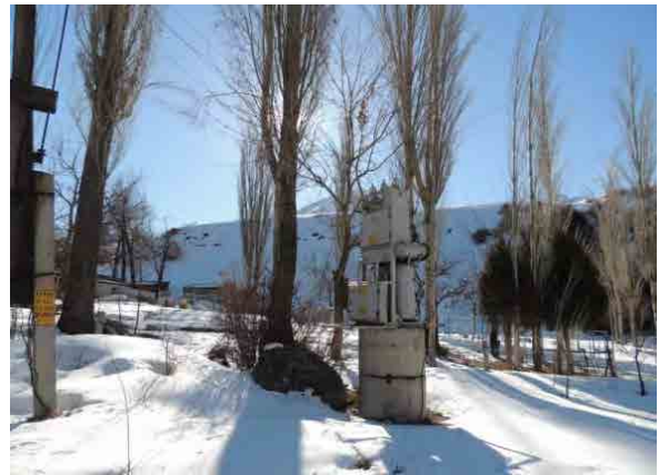
Photo 6-2-52 10/0.4kV Transformer located 2km down the stream of Ysyk-Ata River from Candidate Power Station Location
