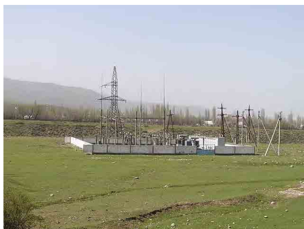
Photo 6-2-90: 35kV Shamsi Substation
