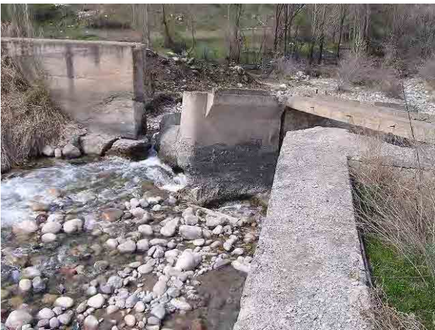
Photo 6-2-66: Damaged Old Intake Weir
