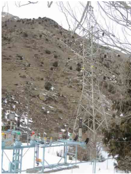
Photo 6-2-77 35kV Distribution Line to Sk-Bulak Substation
