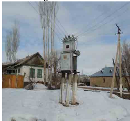
Photo 6-2-71 10/0.4kV Transformer in Bululu Village
