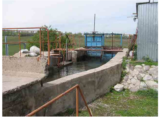
Photo 6-2-107: Headtank for Captive Power
