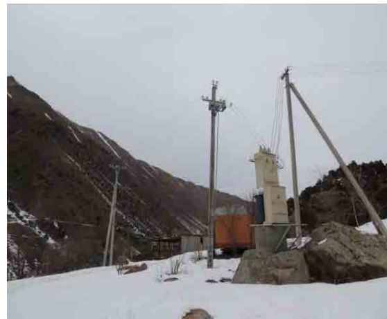
Photo 6-2-80 10/0.4kV Transformer located near the Intake Point
