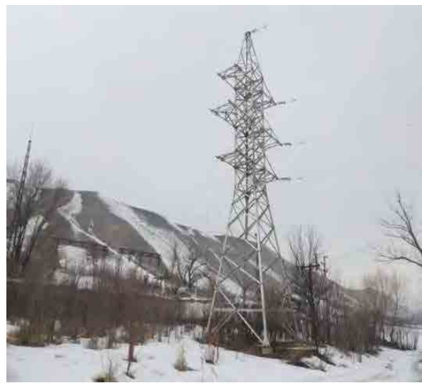
Photo 6-2-69 35kV Distribution Line to Belogorka Substation
