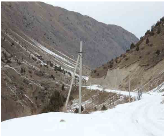
Photo 6-2-79 10kV Distribution Line from Sk-Bulak Substation
