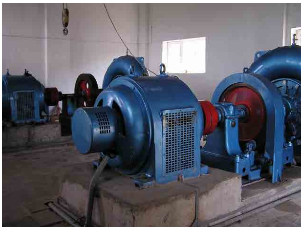
Photo 6-2-110: Generator for Captive Power
