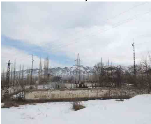
Photo 6-2-70 35/10kV Belogorka Substation
