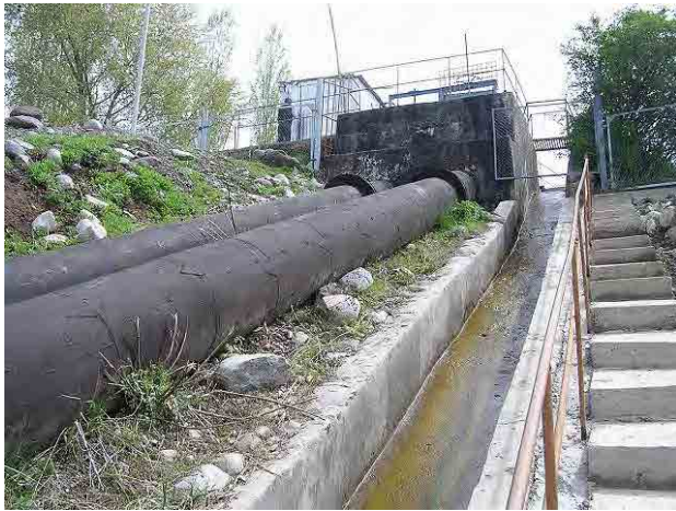
Photo 6-2-108: Penstock for Captive Power
