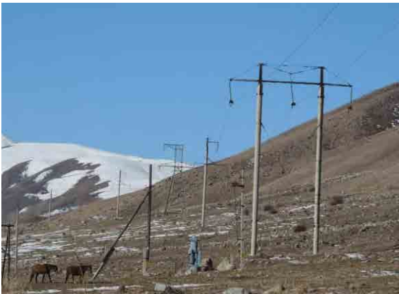
Photo 6-2-51 220kV Ala-Archa – Bystrovka Line
