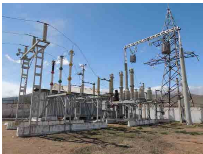
Photo 6-2-100 110/35/10kV Shabdan Substation
