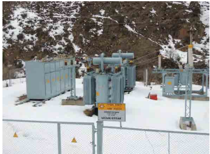
Photo 6-2-78 35/10kV Sk-Bulak Substation
