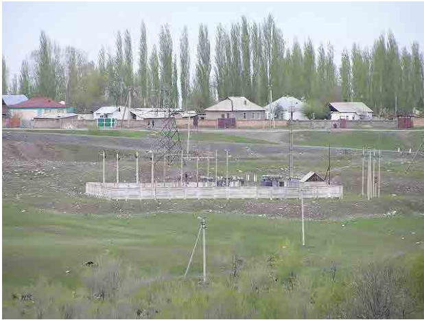
Photo 6-2-112: 35 kV Substation near the Site
