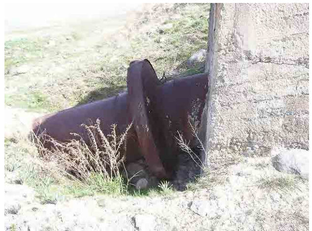
Photo 6-2-57: penstock and Anchor Block
