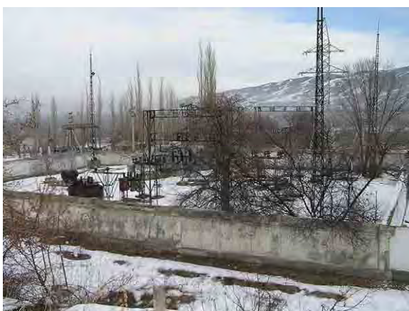
Photo 5-7-11: 35kV Substation adjacent to Powerhouse
