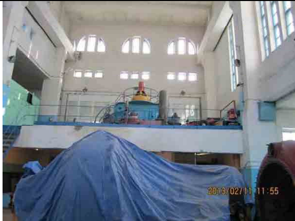
Photo 5-7-15: Inside of Powerhouse
