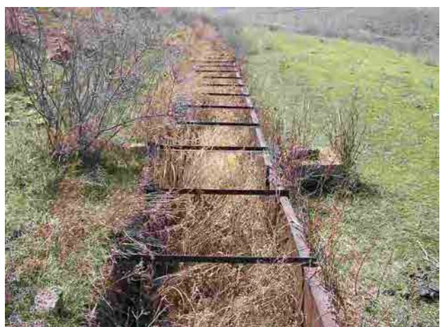
Photo 6-2-34: Headrace (1 m wide, 4mm thick steel plate)
