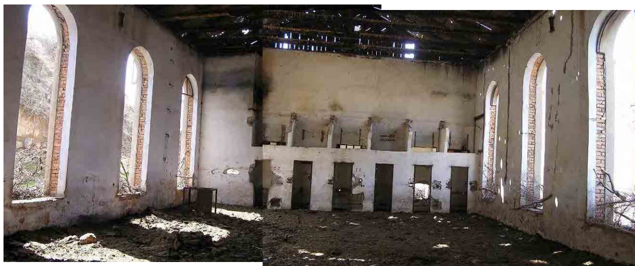
Photo 6-2-23: Inside of Powerhouse
