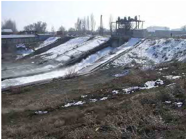
Photo 5-7-12: Bypass Discharge Facility
