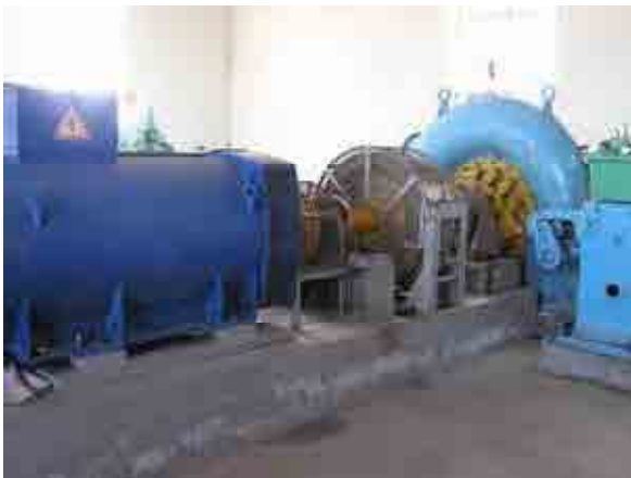
Photo 5-7-5 Inside Powerhouse (Turbine, Generator)
