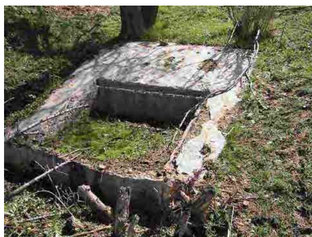
Photo 6-2-25: Anchor Block for Penstock
