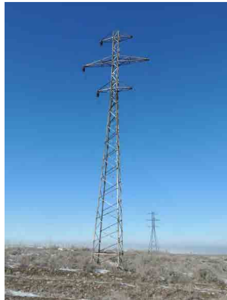
Photo 6-2-18 35kV Koroi - Kegeti Line
