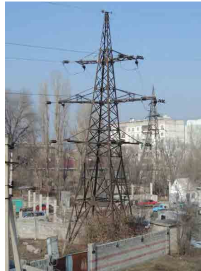
Photo 5-7-18 35kV Distribution Line
