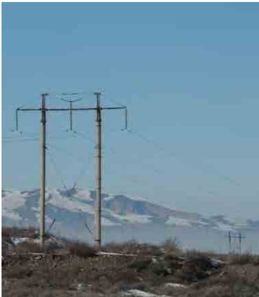
Photo 6-2-17 220kV Ala-Archa – Bystrovka Line
