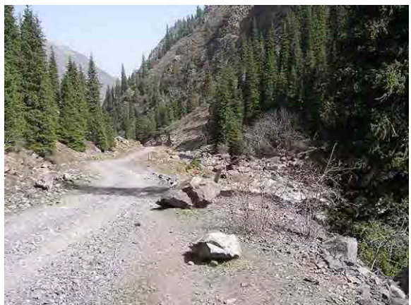
Photo 6-2-6: Fallen Rocks on road between A&B
