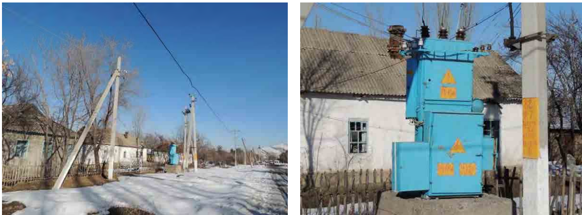
Photo 5-4-1 10kV Distribution Line (Left) and 10/0.4kV Transformer (Right) in Kegeti Village
