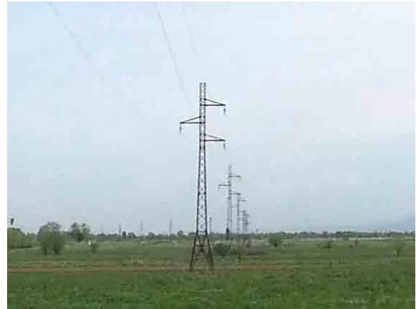
Photo 6-2-45 35kV Distribution Line (Location of the Terminal Substation is unknown)
