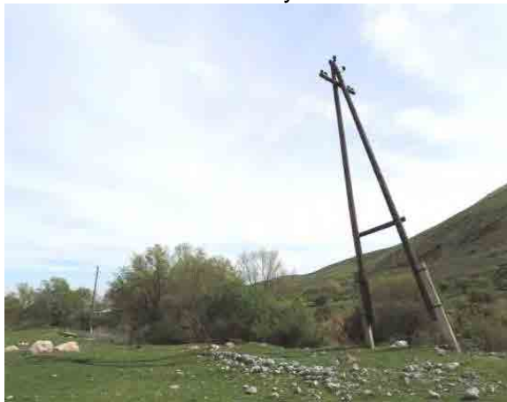
Photo 6-2-46 Terminal Point of Existing 10kV Distribution Line
