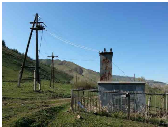
Photo 6-2-19 10/0.4kV Transformer closest to Candidate Power Station Location
