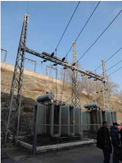
Photo 5-7-17 Step-up Transformer of Power Station (6/35kV)
