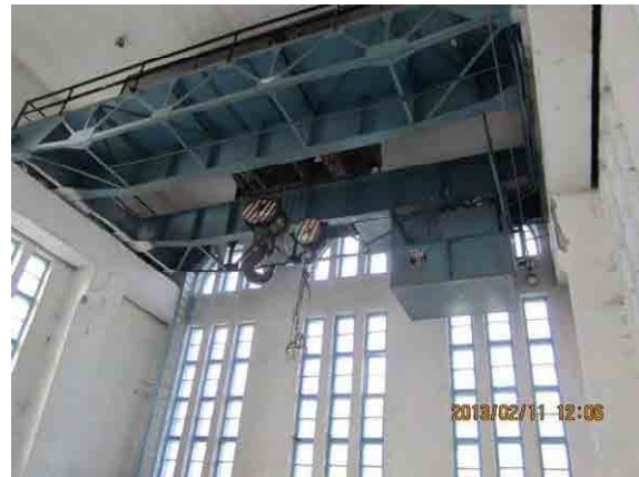
Photo 5-7-16: Overhead Traveling Crane
