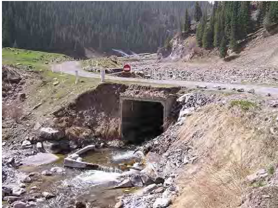
Photo 6-2-1: Road closed point Estimated Q = 0.2 - 0.3 \text{ m}^3/\text{s}
