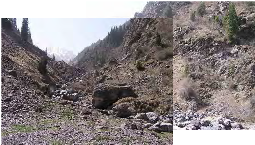
Photo 6-2-10: Steep slope section between B and C (seen from downstream to B)
