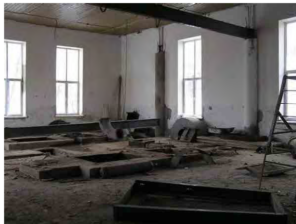
Photo 5-7-10 Inside of Powerhouse
