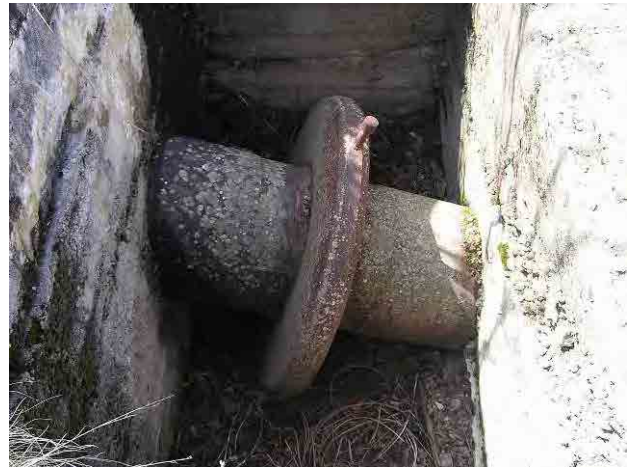
Photo 6-2-27: Penstock ( \Phi 600 mm)
