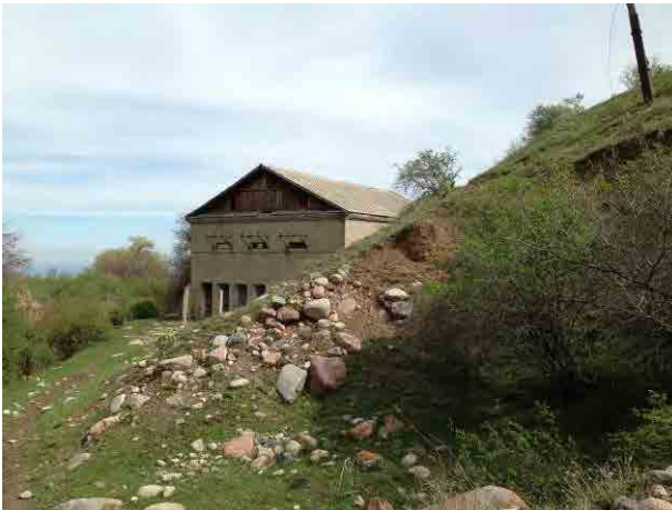
Djardy-Kainda: The roof of the old power house is made of corrugated slate which may contain asbestos.
