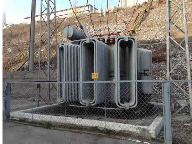
Transformer in an operating small hydropower station: The possibility is low that PCBs, hazardous substances, are contained at high concentration because the oil is exchanged periodically.
