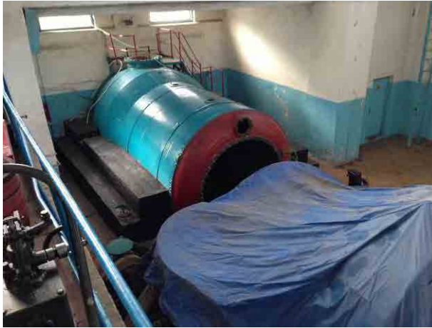
Lebedinovka: Water turbine generator left unrepaired. Appropriate actions like recycling of metals shall be taken in the rehabilitation.
