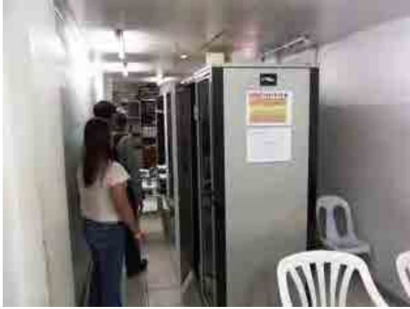
Allocation of racks for traffic signal control
