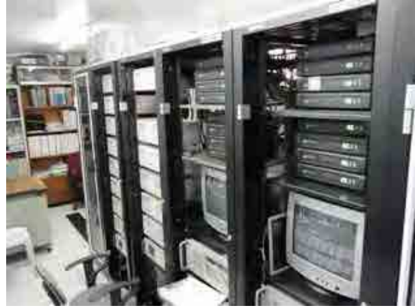
Allocation of racks for traffic signal control
