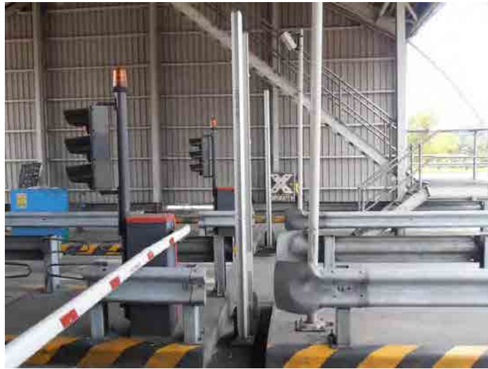
FIGURE 6.2-11 TRAFFIC CONTROL GATE
