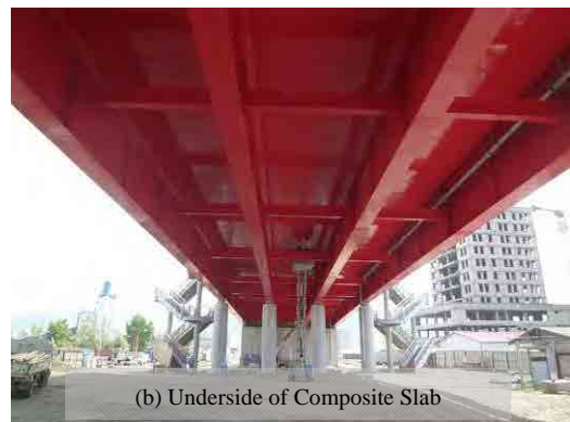
Figure 7.5.7 Bottom of Slab
