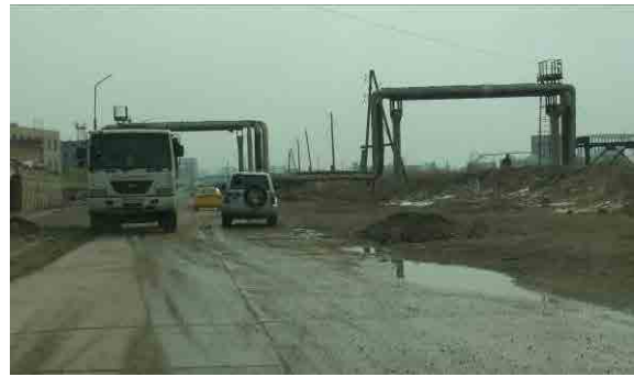
Figure 6.4.2 Hot-water Pipes around STA. 0+440
