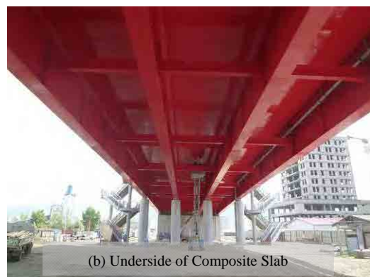
Figure 7.5.7 Bottom of Slab
