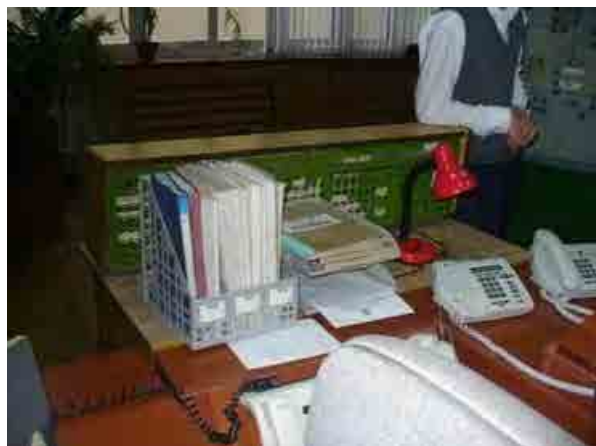
Tashkent-Djizak Section: Operating Switches Panel
