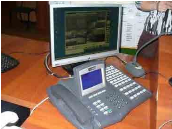
Tukimachi-Angren Section: Display of SCADA and Telephone System for Power Supply Control
