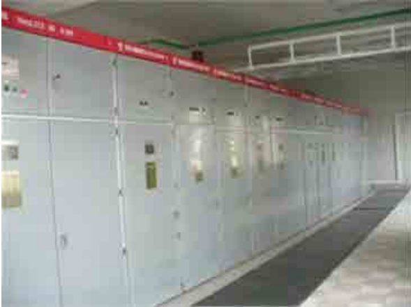
Extra High Tension Distribution Panel
