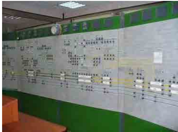
Tashkent-Djizak Section: Indicator Panel of the Power Supply System
