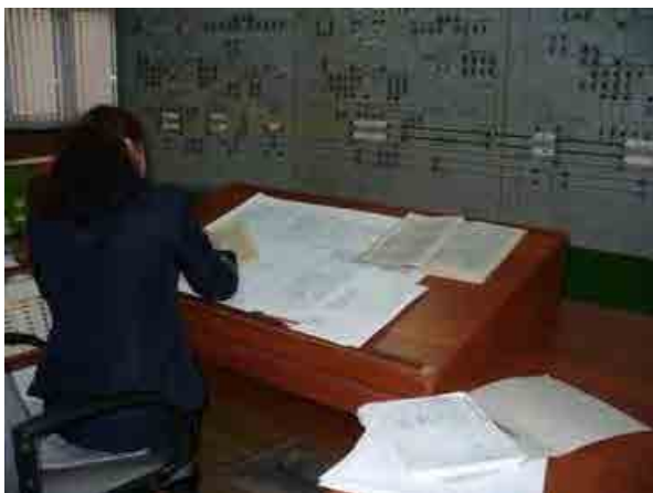
Tashkent-Djizak Section: Operator Console
