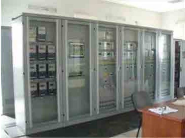
Protective Relay Panel
