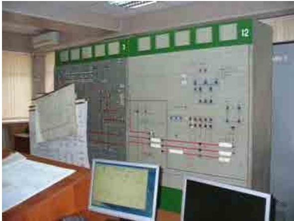
Tukimachi-Angren Section: Indicator Panel of the Power Supply System
