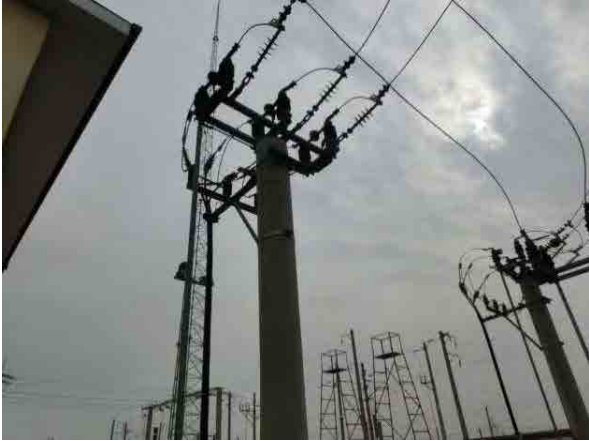
Extra High Tension Distribution Line
