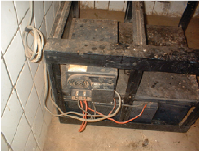
Figure 4.9.5: The Inverter and battery back up
