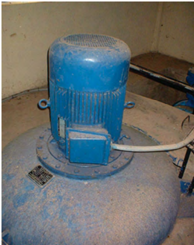
Figure 4.10.3: The Turbine/Generator set
