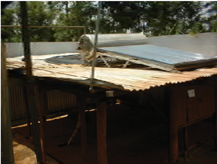
Figure 4.7.5: Digester Solar water heating system
