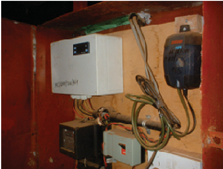
Figure 4.6.8: Power Distribution Board
