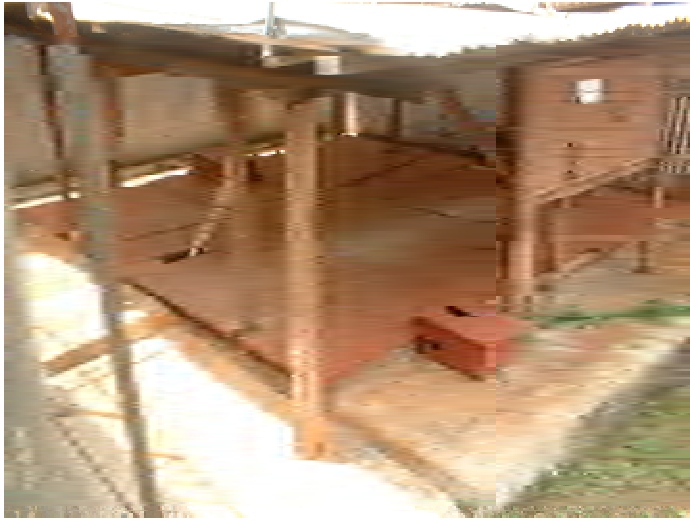
Figure 4.7.4: Underground Digester tank
