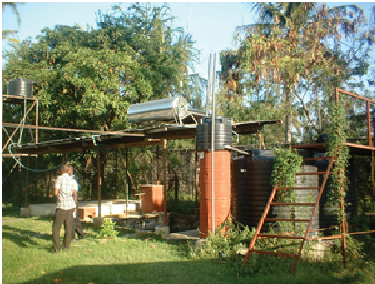
Figure 4.8.1: Wema Centre Biogas Plant
