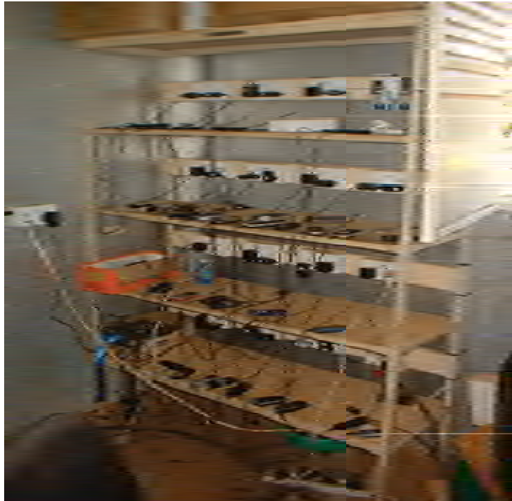
Figure 4.3.5: Charging station for mobile phones and LED lamps
