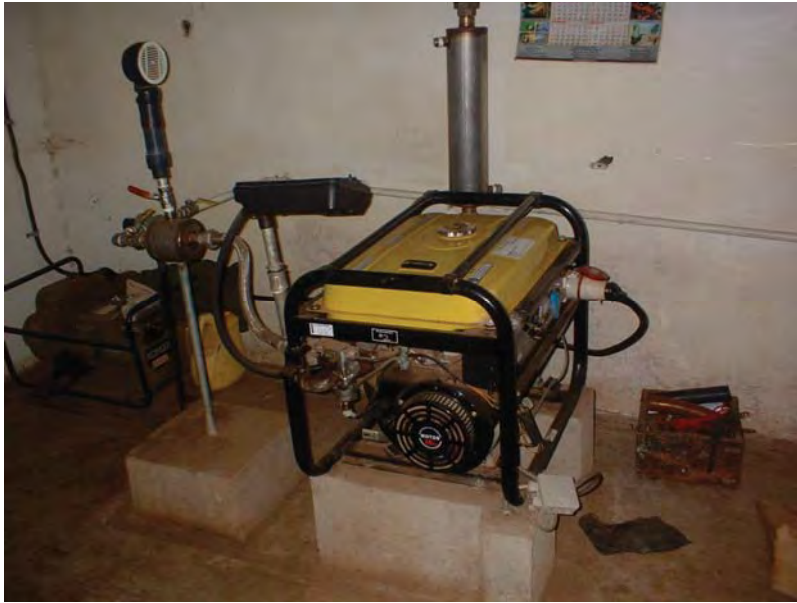
Figure 4.4.6: The 9 kW Powermac Biogas Electric Generator
