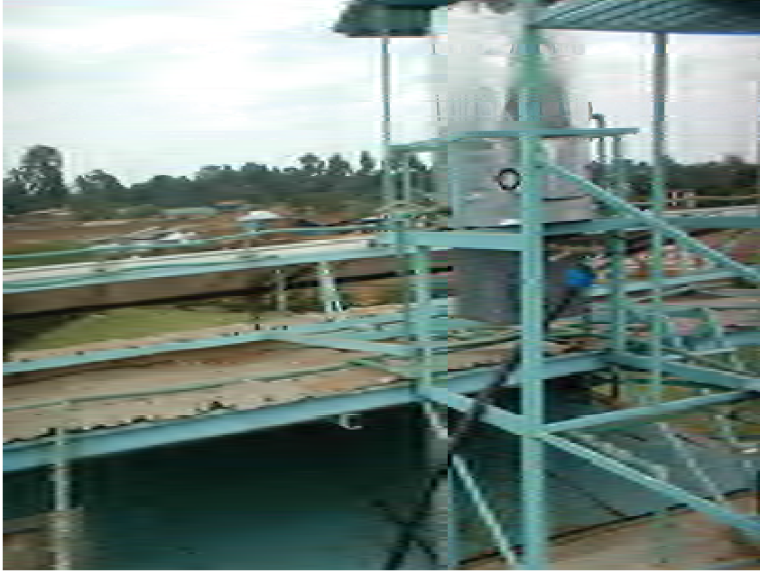
Figure 4.4.4: Digester Solar Heating System
