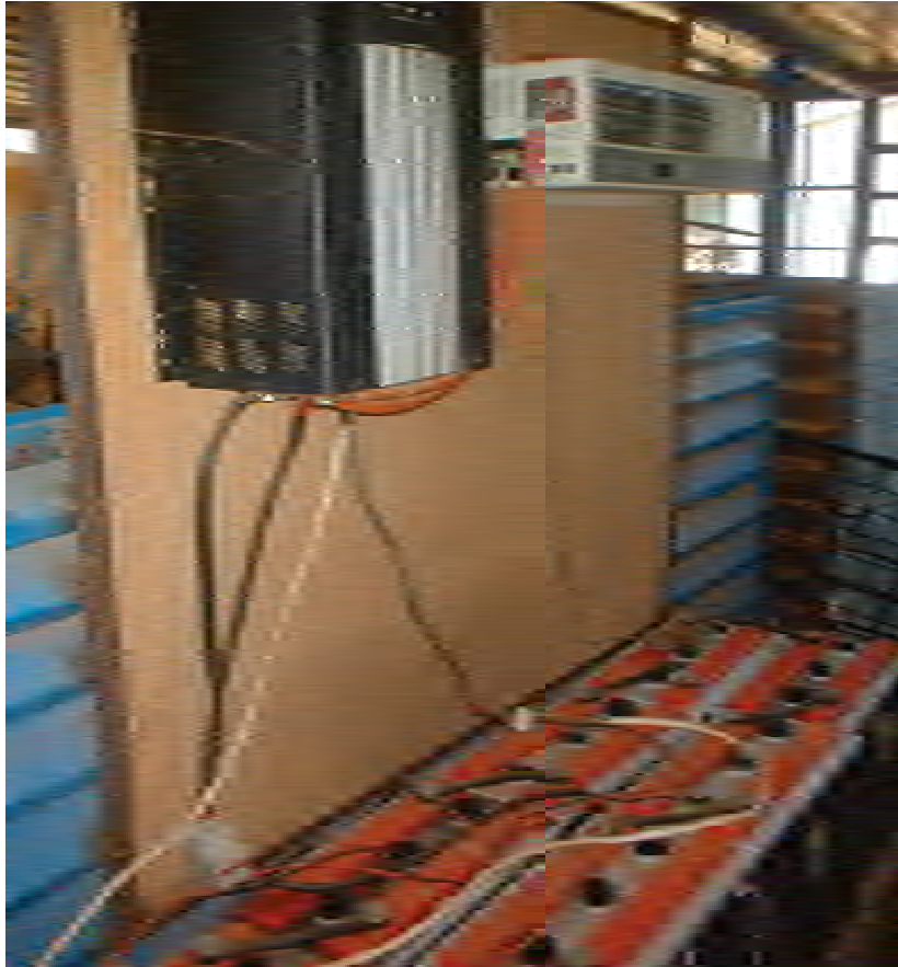
Figure 4.3.3: Uhuru CPC system components: Optisolar Controller ,Inverter, storage batteries
