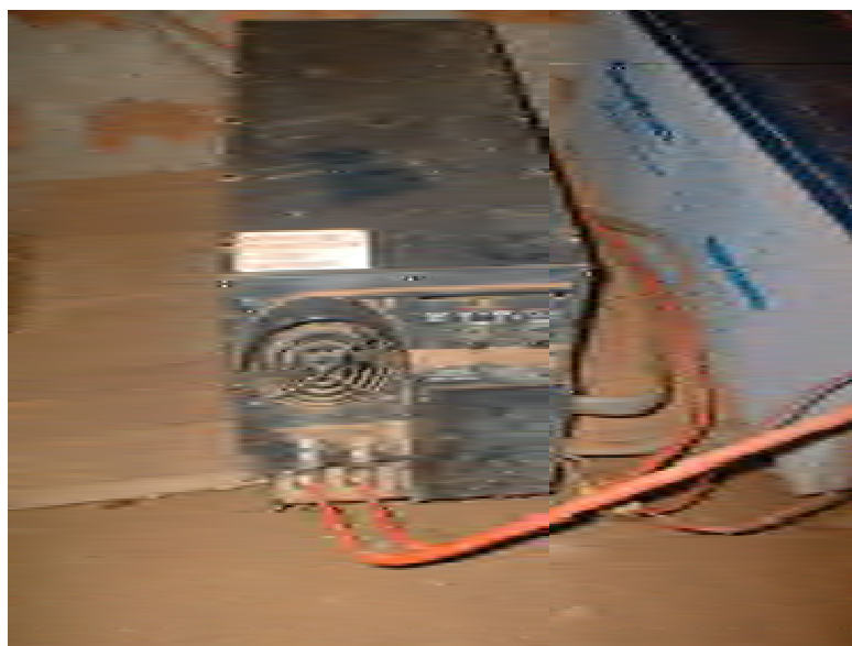
Figure 4.6.7: Backup power Inverter/Charger and Battery
