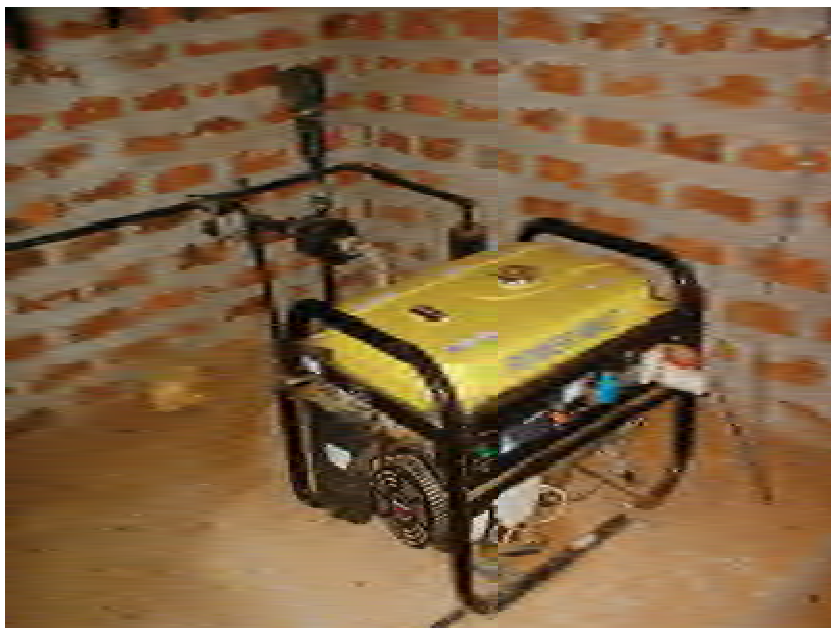
Figure 4.6.6: The 9 kW Powermac Biogas Electric Generator
