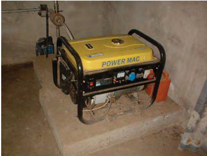
Figure 4.5.6: The 9 kW Powermac Biogas Electric Generator
