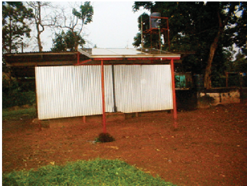
Figure 4.6.5: Digester Solar Heating System
