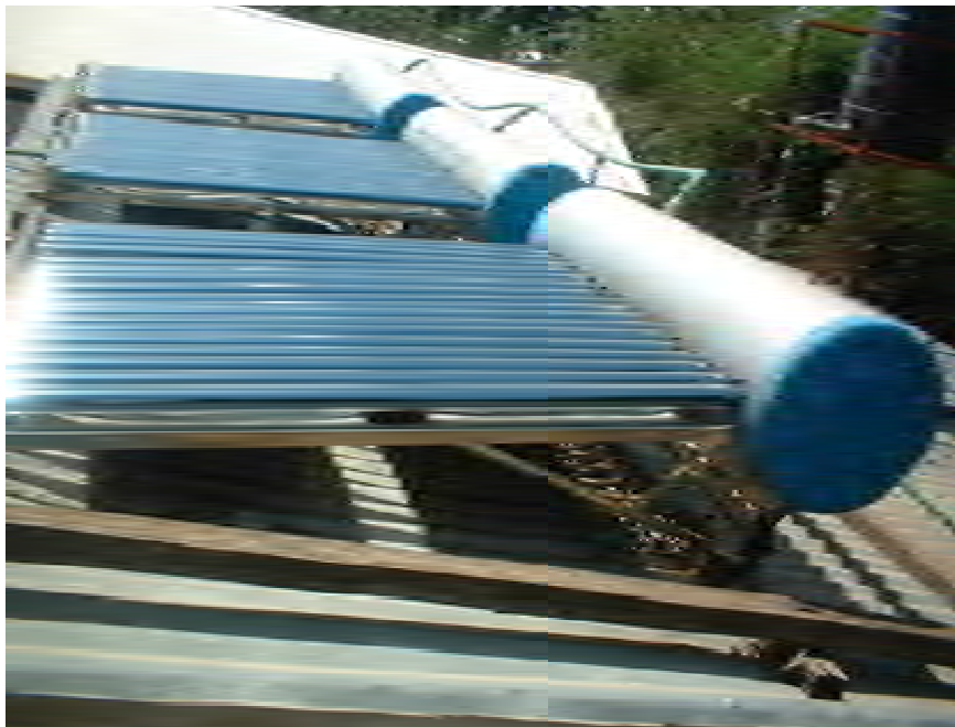
Figure 4.5.5: Digester Solar Heating System
