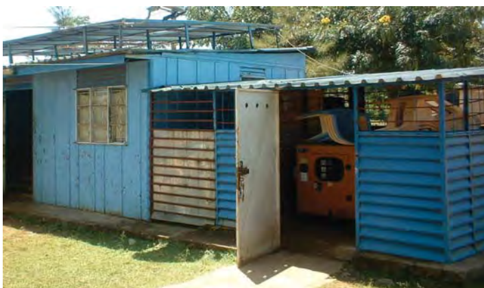
Figure 4.3.4: Uhuru CPC system components: Solar array on container roof and a section of 8kW SVO Generator in the power house.
