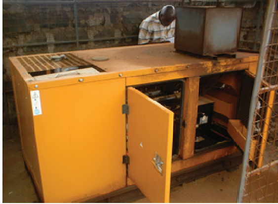
Figure 4.1.4: CPC System Components: The Duo-Fuel Generator with Rencon's John Kyalo taking down the details
