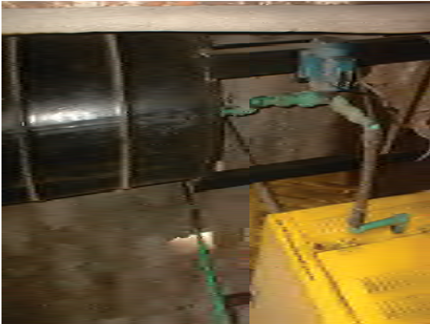
Figure 4.2.5: Improvised Cooling system
