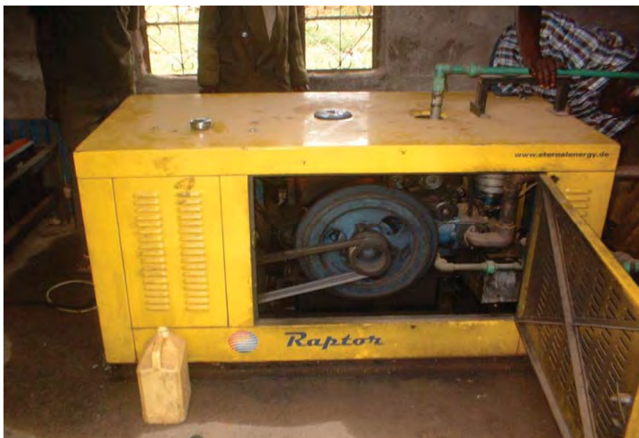
Figure 4.2.4: The 8 kW Raptor SVO Generator
