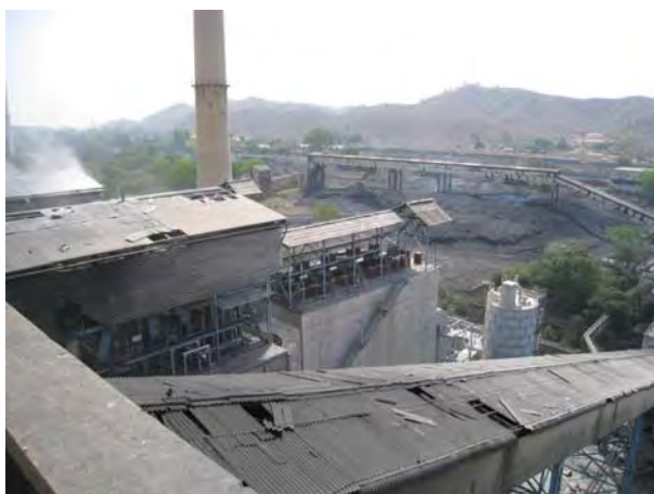
Boiler, ESP & Coal Yard
