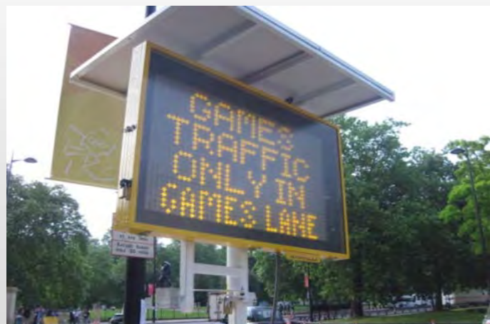
VMS – Lane Management
