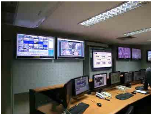
Photo: Control Center (AGETRANSP)
