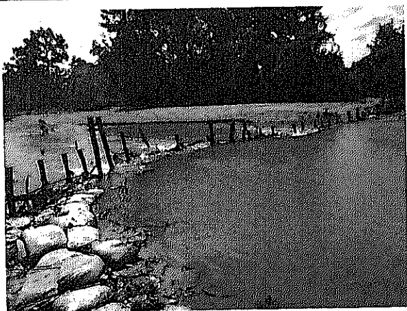
Temporary weir for Daun Pue Intake made with sand bags and wooden material
