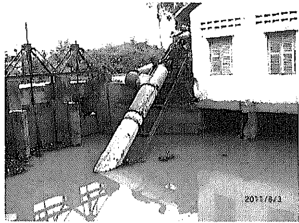
Existing intake and pump station at Tonle Bati Lake (intake gates are heavily deteriorated and pump capacity is much less than required one)
