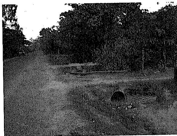
Pipe culvert on main canal (to be replaced)
