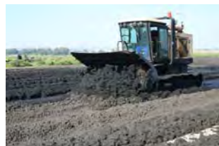
Sludge Turn-over & Drying, Johannesburg
