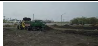
Solar Drying, Nong Khaem WWTP, Bangkok
