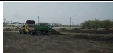
Solar Drying, Nong Khaem WWTP, Bangkok
