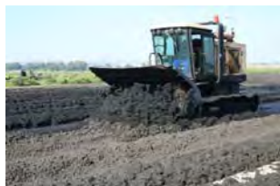
Sludge Turn-over & Drying, Johannesburg
