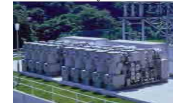
Gas Insulated Substation
