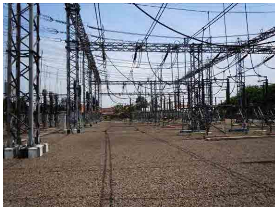
Photo Switchyard at Cikupa Substation
