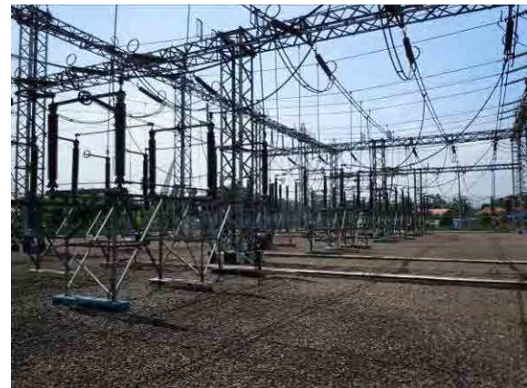
Photo Switchyard at Cikupa Substation
