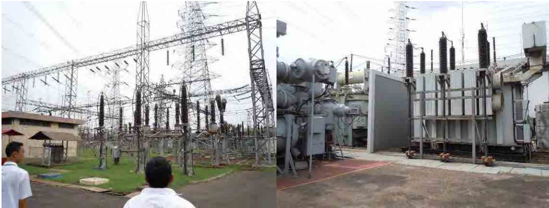
Figure 5.26 Cable Interconnection at Plogadung Substation
