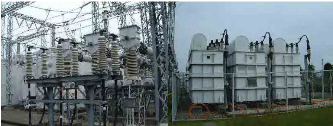
Figure 5.27 Example of Cable Usage for TEPCO's Capacitor Banks
