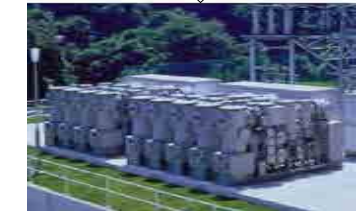
Gas Insulated Substation
