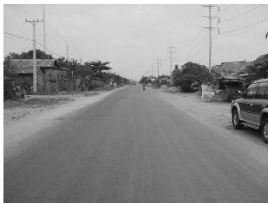
Photo 4.1-2 Roadside Higher than Road Surface without Drainage
