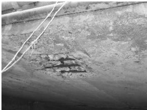
Photo 4.1-3 Damage of Br20
