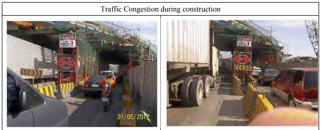
Above picture is shown for shoring/scaffolding of voided slab during construction for similar project. Traffic lane become 2 lanes from existing 3 lanes and cause of heavy traffic jam during construction
