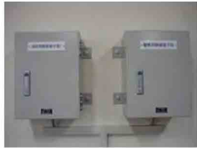
Radio repeat facilities
