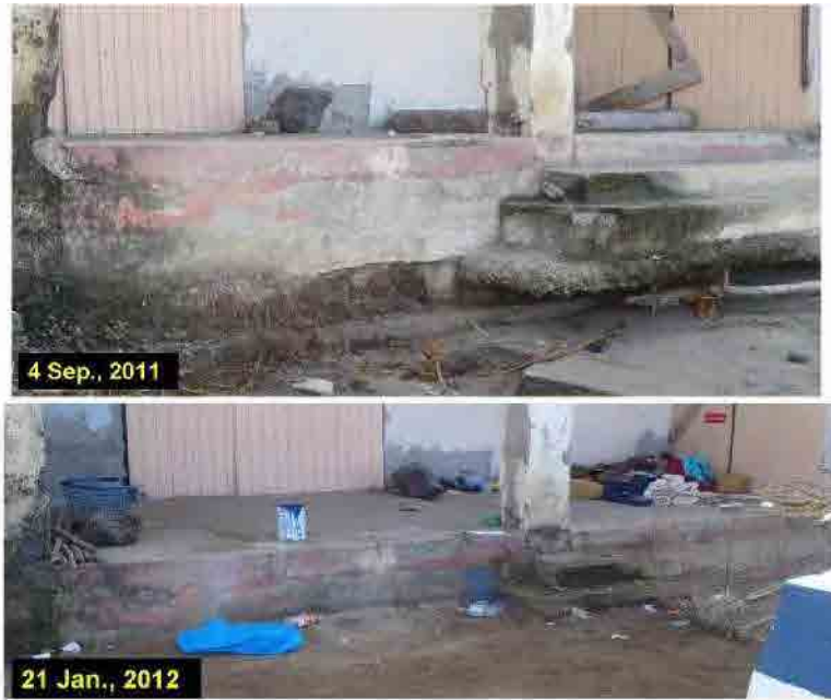
Figure 3-3-1-12 Scour at the base of Community Center
