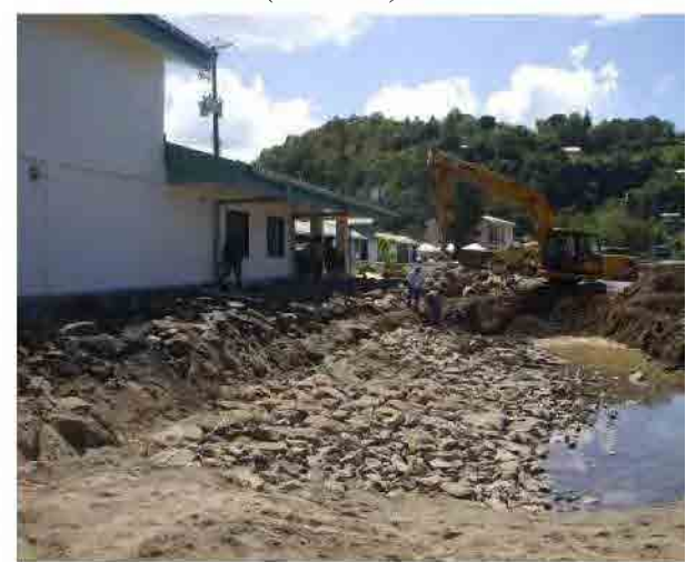
Photo-28 Recovering of rubble stones in front of Fisheries Complex (2013/2/27)
