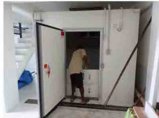
Ice strage room
