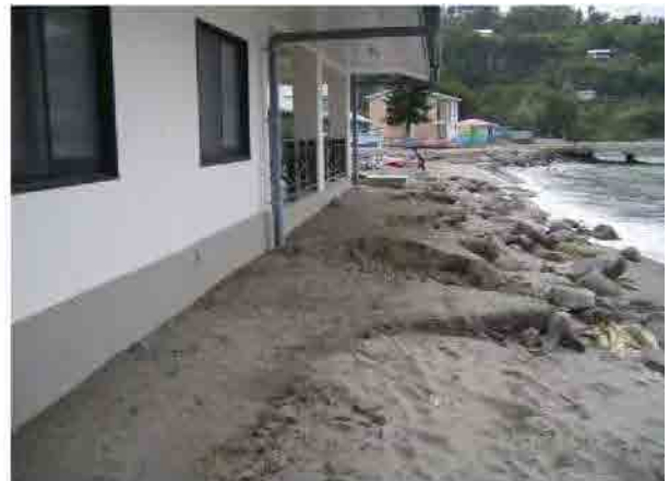
Photo-8 Foreshore condition of Fisheries Complex after passing Hurricane Tomas (2010/11/02)
