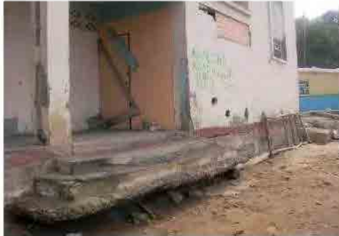
Subsidence in front of the Community Center at one year inspection; Feb. 08, 2011
