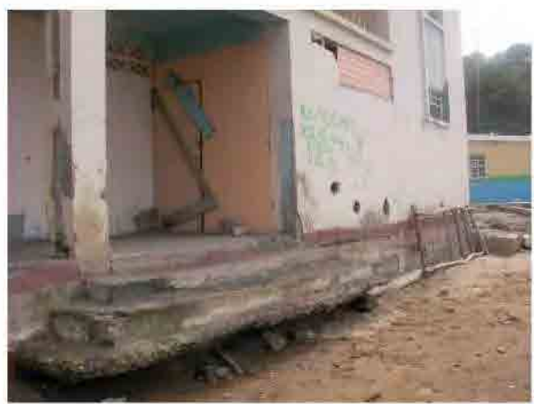
Photo-10 Erosion condition of Community Center at one year inspection (2011/02/28)
