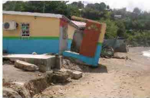
Old warehouse of the Fisheries Cooperative (partially collapse of building) at one year inspection; Feb. 08, 2011
