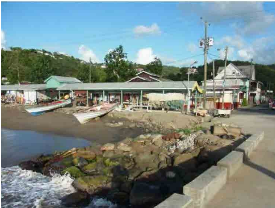
Photo 2-2-3-11 Beach situation of rubble stones in base part of the jetty
