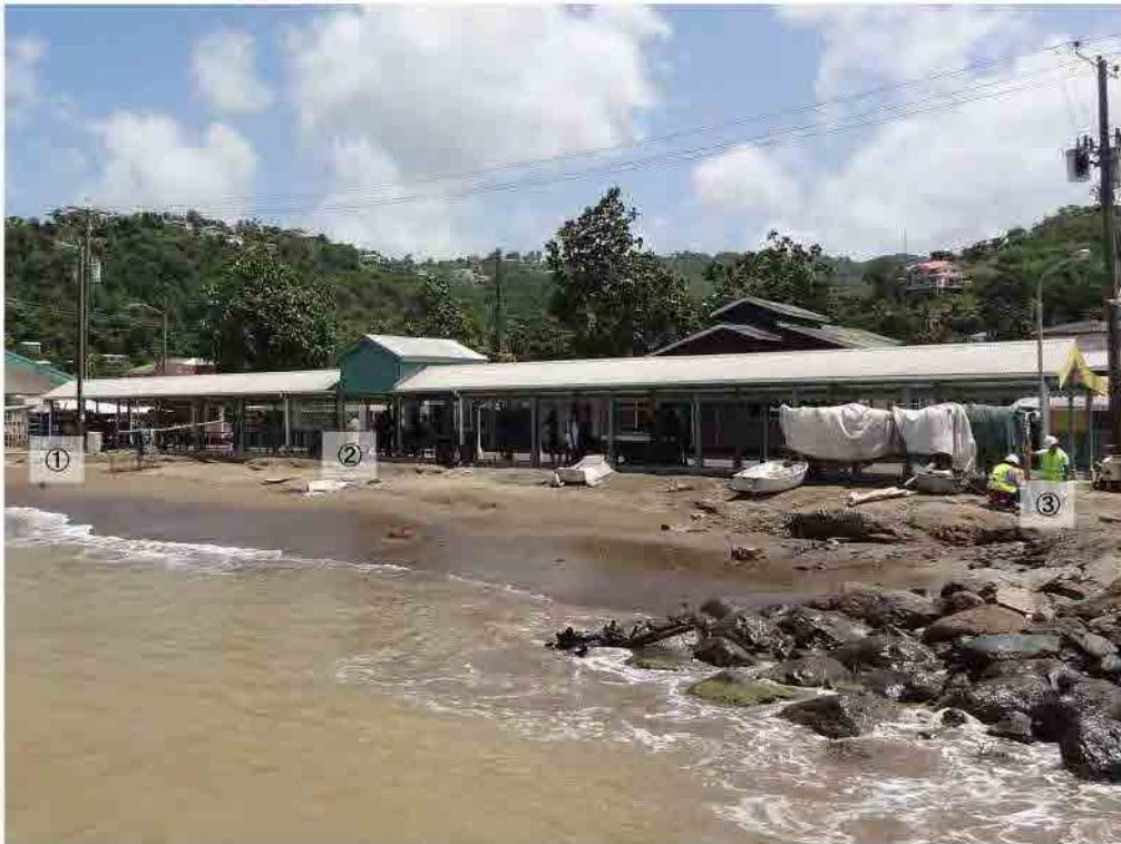
Photo 2-1-2-6 Grand subsidence situation of Fisheries Complex (2)
