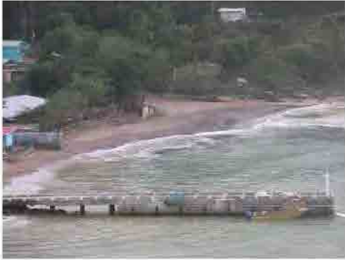
Subsidence and recession of shoreline in North side beach from the Jetty
