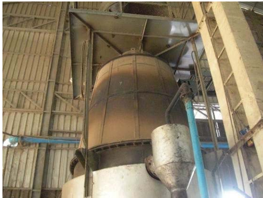
Rice husk gasification power plant (reacting furnace)
