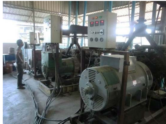
Rice husk gasification power plant (gas engine)
