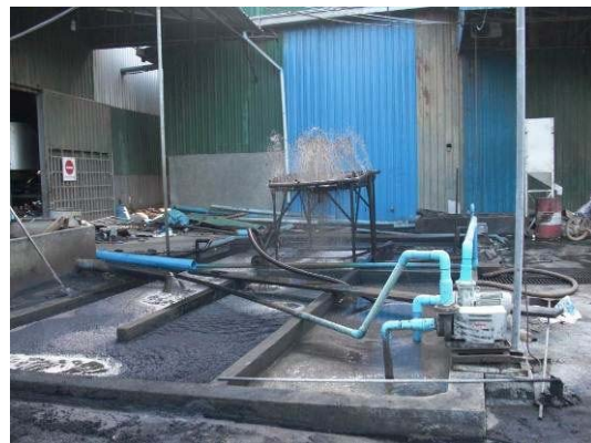
Drainage water treatment equipment of a rice husk gasification power plant
