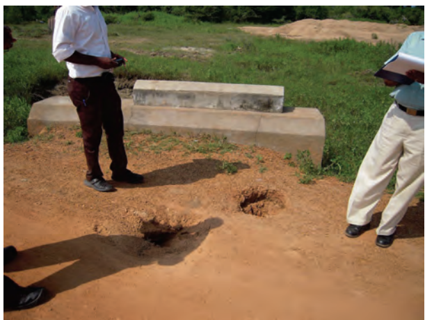
Theththavaady Road Flood Damage (3)
