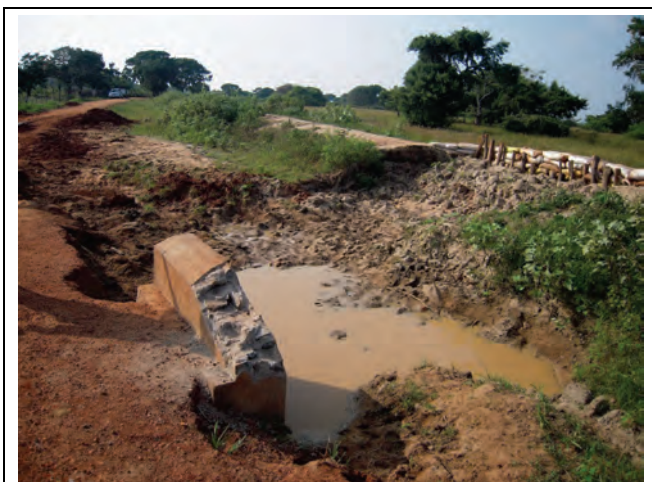
Pali Aru Tank Breached and Road Erosion
