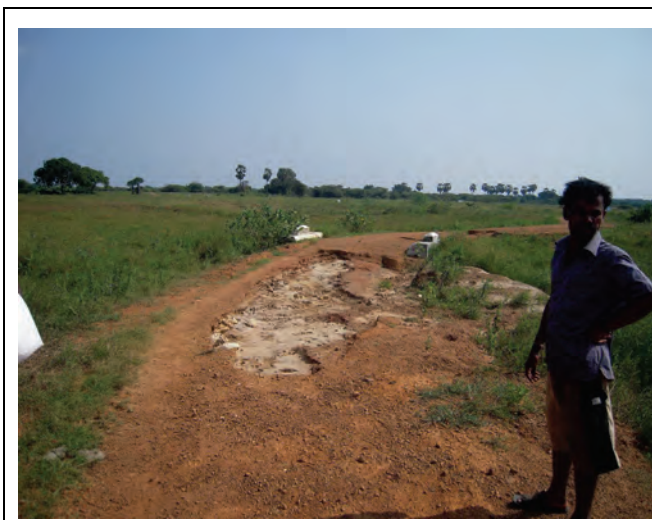
Theththavaady Road Flood Damage (5)
