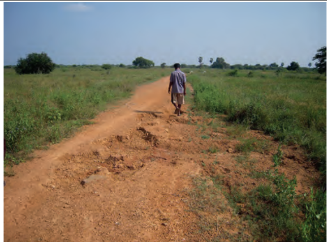
Theththavaady Road Flood Damage (4)
