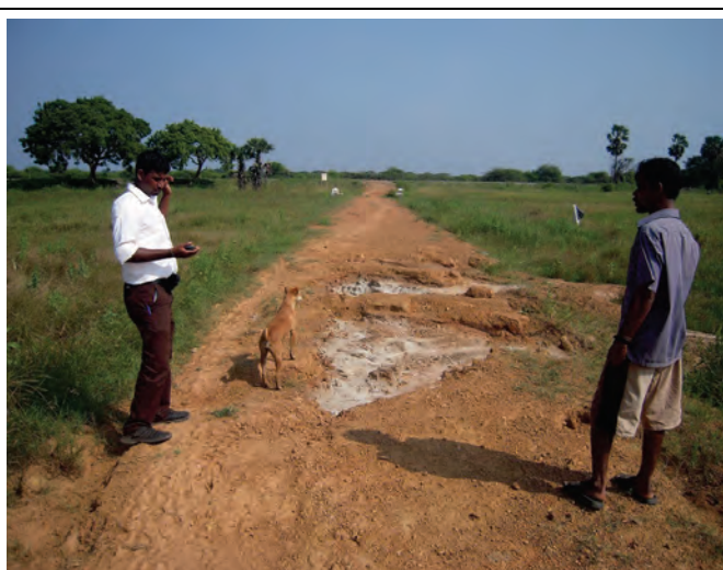
Theththavaady Road Flood Damage (6)
