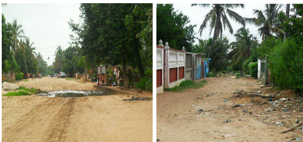
Figure 29: State of the wider roads closer to the EN1
