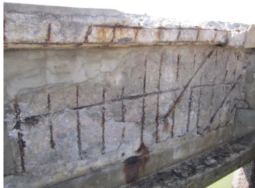
Conspicuous exposure of reinforcing bars
