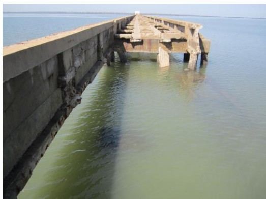
Intake bridge for old Maputo coal-fired power plant (partially damaged) (Source: JICA Study Team)
