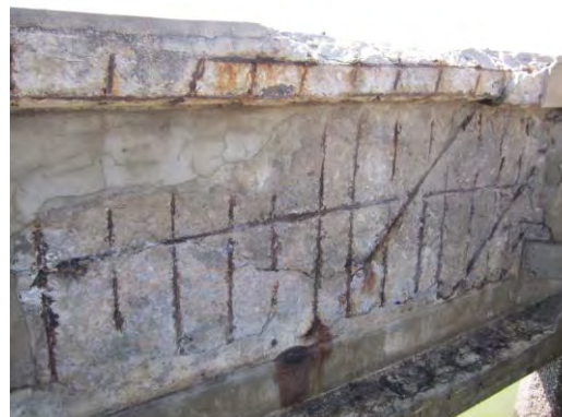
Conspicuous exposure of reinforcing bars
