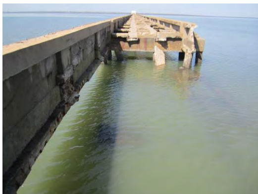
Intake bridge for old Maputo coal-fired power plant (partially damaged) (Source: JICA Study Team)
