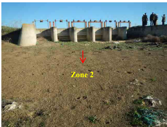
Figure 3-23 Overflow Weir (Zone 3 to Zone 2) with Gate
