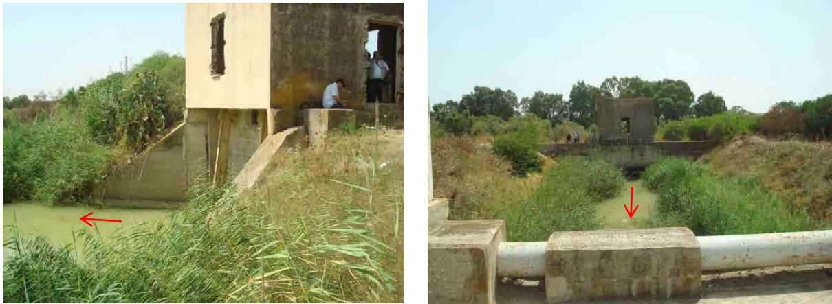
Figure 3-20 El Mabtouh Retarding Basin Diversion Channel Confluence with Mejerda River and Gate Facilities
