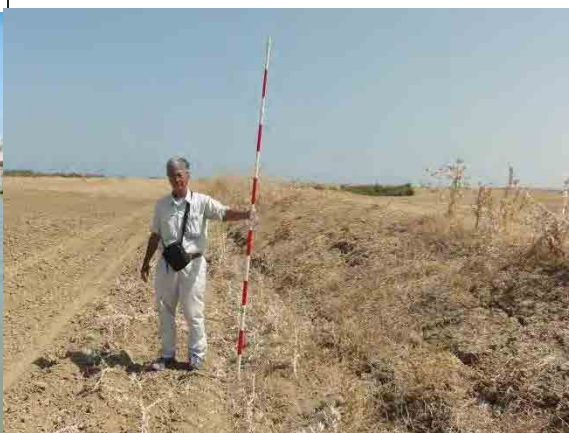
28. Delta bridge right bank downstream embankment flow situation (2012.09)
