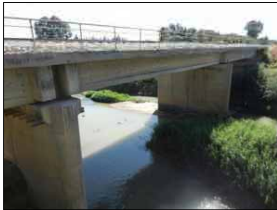
Figure 6.3-9 Current Status of Jedeida Railway Bridge (Aug., 2012)
