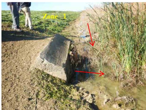
Figure 3-27 Flap Gate at Outlet of Discharge Sluiceway
