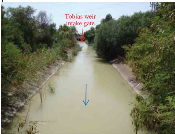
26. Water conduit from the Tobias weir (2012.08)
