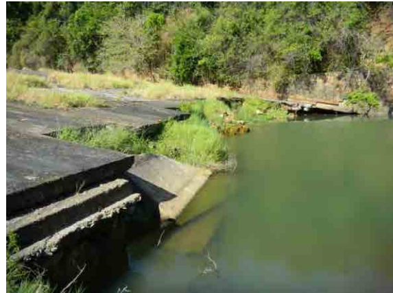
Broken spillway (Trincomalee)
