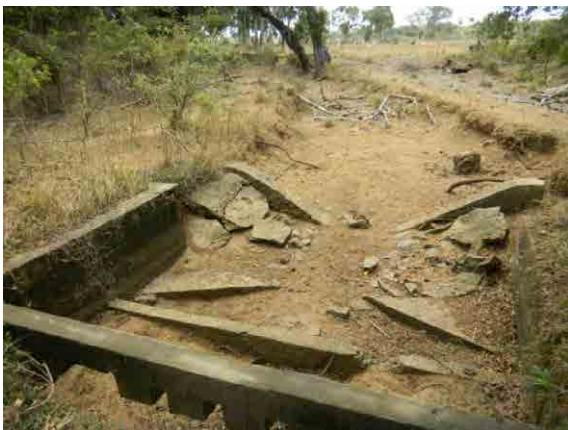
Broken Outlet (Trincomalee)
