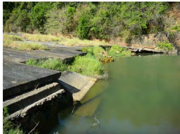
Broken spillway (Trincomalee)
