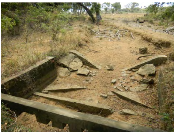
Broken Outlet (Trincomalee)
