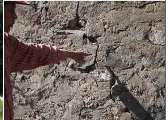
Crack of retaining wall on part slope on road
