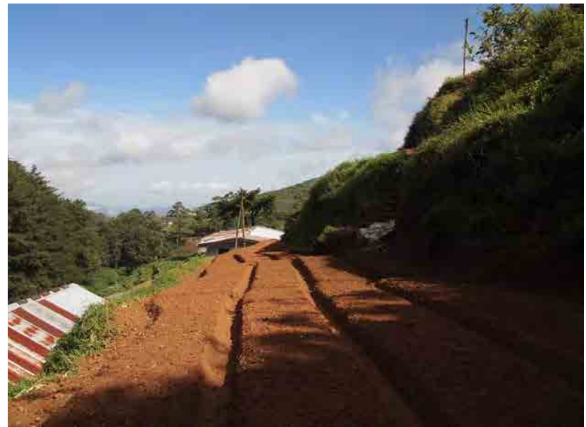
Condition of slope, house under slope
