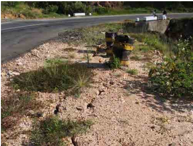
Tension cracks along the shoulder of the road at the beginning side.
