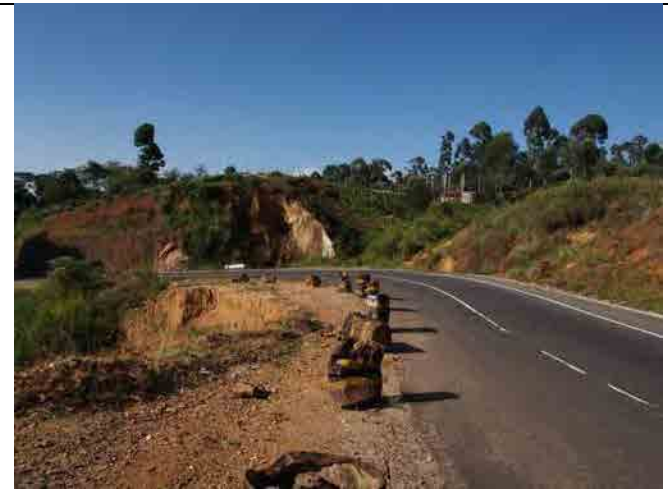
Condition of the road around the head scarp at the ending side.
