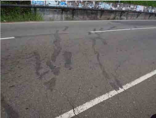
Cracks appeared on the road surface. Cracks seem to follow the shape of a head scarp under the pavement.
