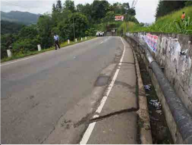
Damage on the road at the middle of the landslide
