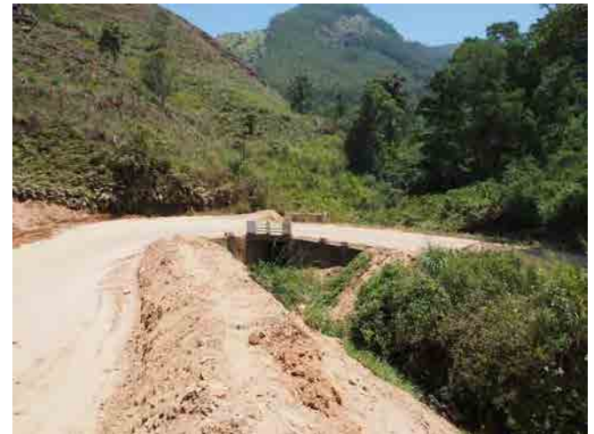
The bridge and the cleaned up debris. Amount of the debris is so big that the river course is about to be closed.
