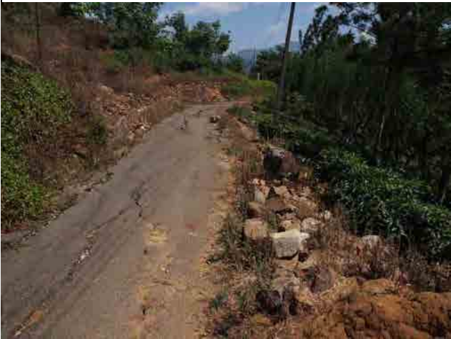
Cracks at the middle of landslide.
