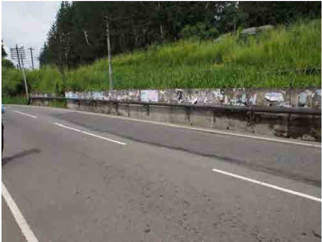
Retaining wall along the road. After the construction of this retaining wall, landslide of upper slope was said to be eased.
