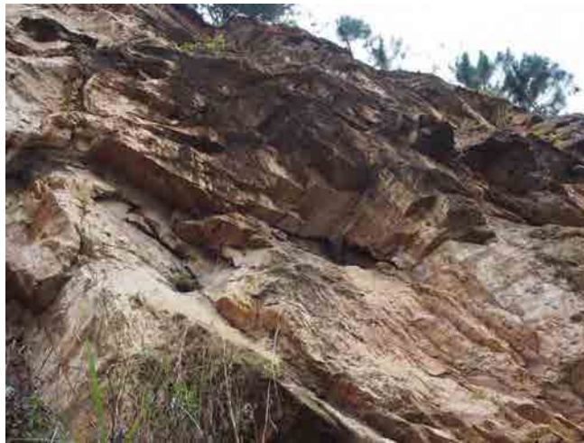
With foliation plunging to the slope, sheeting joints can form slip surfaces for rock slides.
