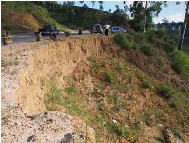
Headscarp along the road shoulder at the ending side
