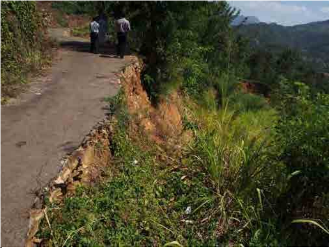
At the middle of the landslide. A head scarp of a divided landslide developed along the paved road.
