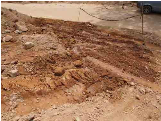
At the toe of the landslide, seepage of water was confirmed
