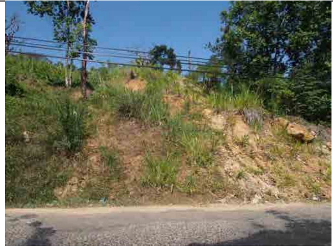
Toe of the landslide. Debris from the landslide accumulated and closed the road when the landslide was activated.
