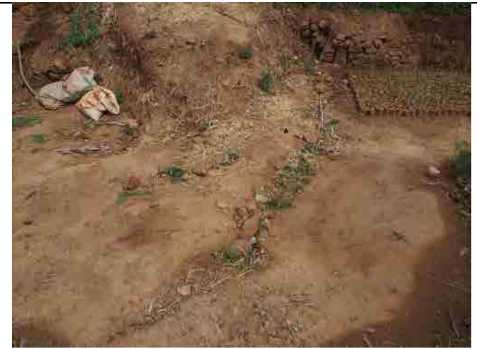
Open cracks seen at the terraces on the upper slope.
