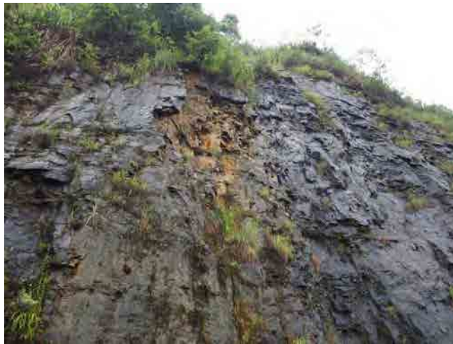
Traces of rock fall or minor rock slides which occurred recently. The height from the road is around 30 meters.
