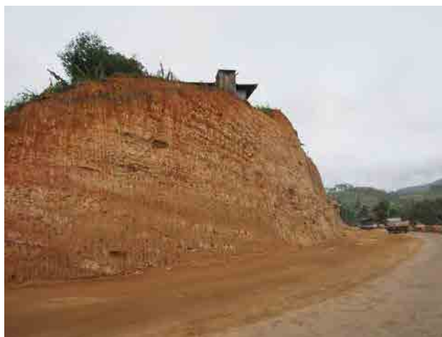
Figure 2-16: Typical Cutting Slope, Too Steep, No Drainage
