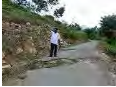
vi) A cracked road, Badulla
