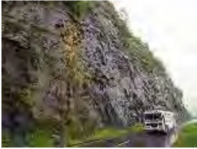
i) Soaring escarpment with fresh traces of collapse at National Road (NR) A005
