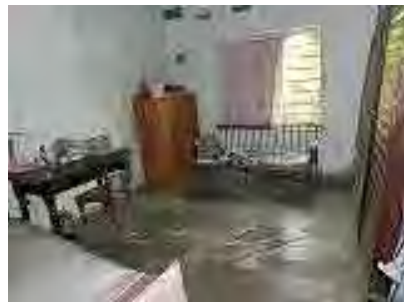
vii) A cracked house, Badulla
