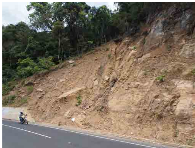
Figure 2-12: Example of Slope Failure
