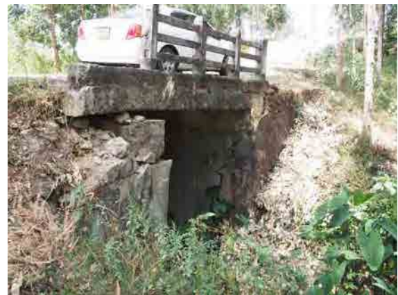
(Crack on the abutment of the small bridge at Km 70)
