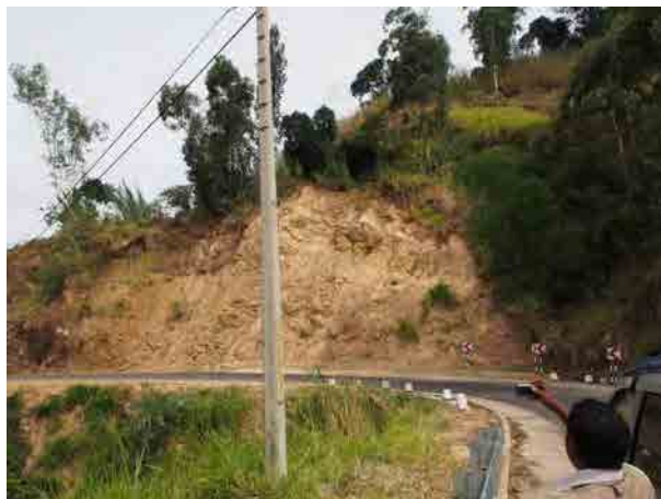
Figure 4-4: Slope failure of A005-091 (Full view)
