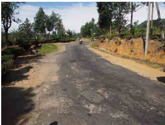
(Subsidence of pavement on B413)
