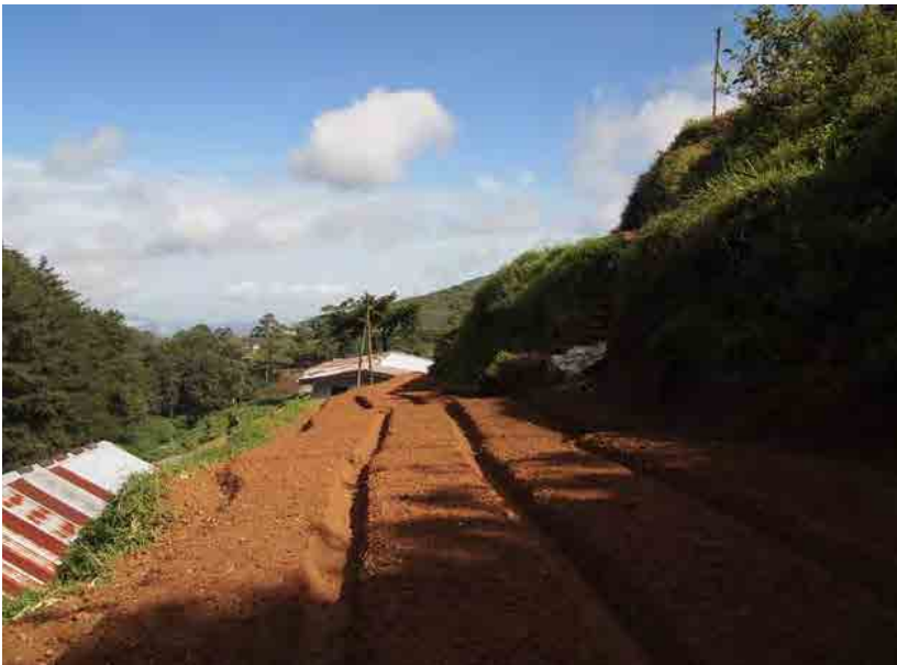
Condition of slope, house under slope
