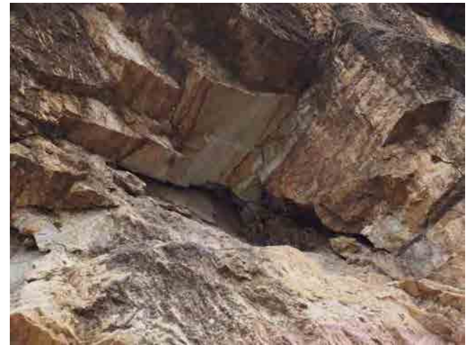
Close up view of the left. The sheeting joints have some aperture, making a rock mass apart from the out crop.
