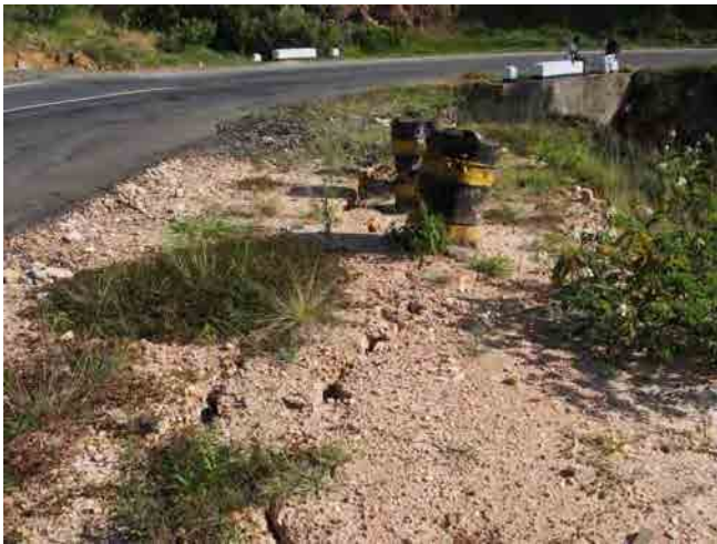
Tension cracks along the shoulder of the road at the beginning side.
