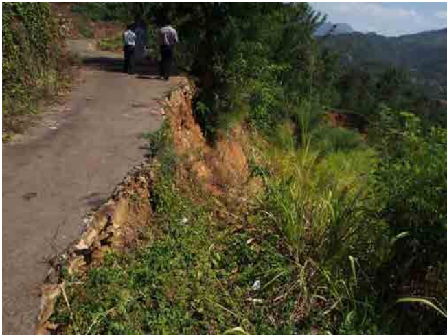
At the middle of the landslide. A head scarp of a divided landslide developed along the paved road.
