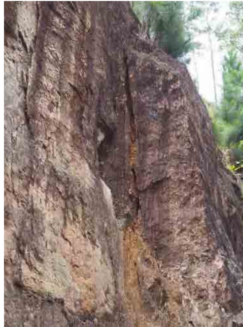
Condition of the slope, open cracks developed behind the rock mass almost perpendicularly.
