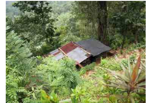
Condition of slope, house under slope
