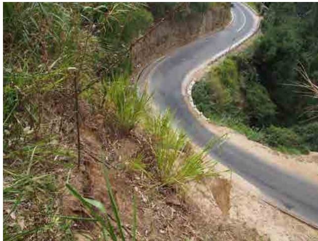
Seen from the shoulder of the failure
