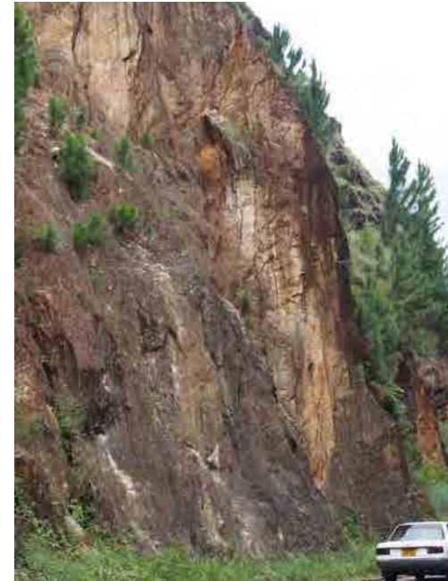
Condition of the slope, Rock slide and rock fall are anticipated. Toppling may occur under certain condition.
