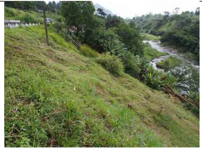
Condition of the lower part of the landslide.
