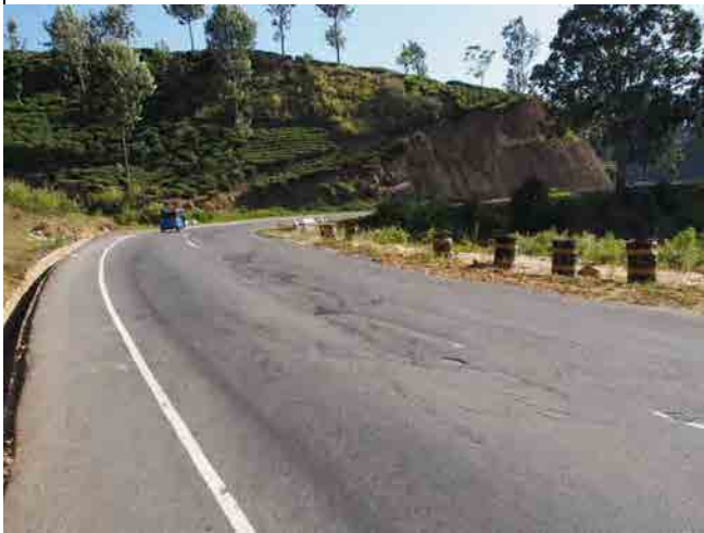
Subsidence on the road at the beginning side.
