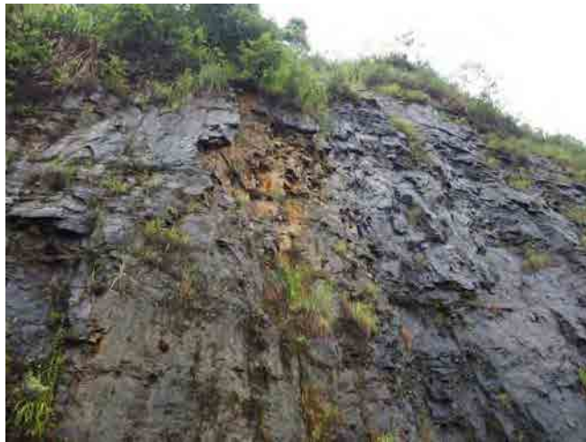
Traces of rock fall or minor rock slides which occurred recently. The height from the road is around 30 meters.
