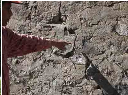
Crack of retaining wall on part slope on road
