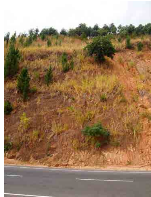
Condition of slope, the slope on the start side is a slope of a steady sedimentary rock
