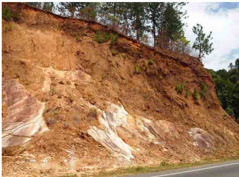
Condition of slope, a loose sedimentary soil is recorded on the base rock.
