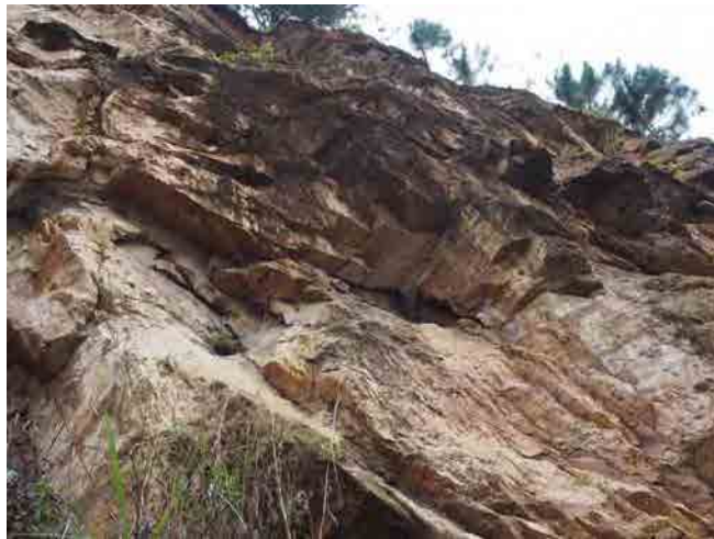
With foliation plunging to the slope, sheeting joints can form slip surfaces for rock slides.
