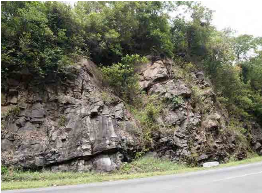
Condition of slope, there are a lot of cracks and floatstones.
