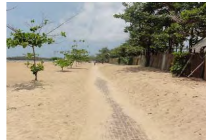
Walkway almost covered by the sand (Nusa Dua)
