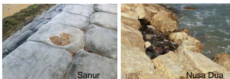
Photo 2.2.2 Damages to Coastal Facilities
