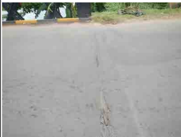
Damage of expansion device Colombo(B388- 2/5)
