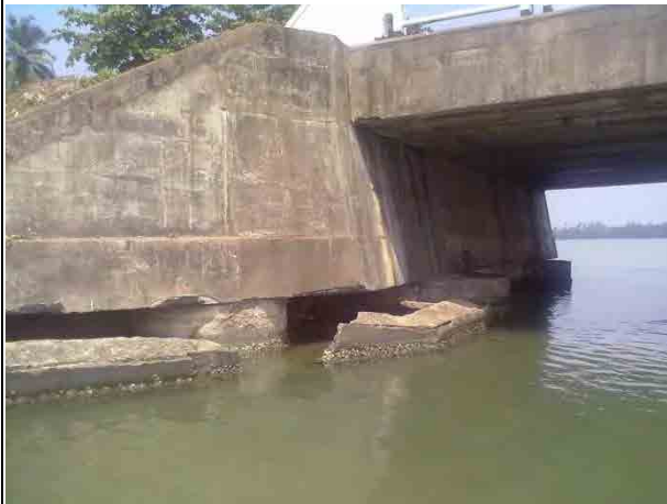
Collapse of abutment Kalutara(AA002- 7/1)
