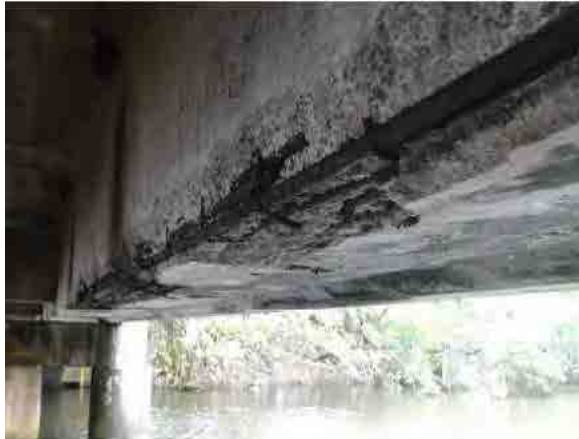
Rebar exposure and corrosion of the concrete girder Kalutara(AA002- 31/3)
