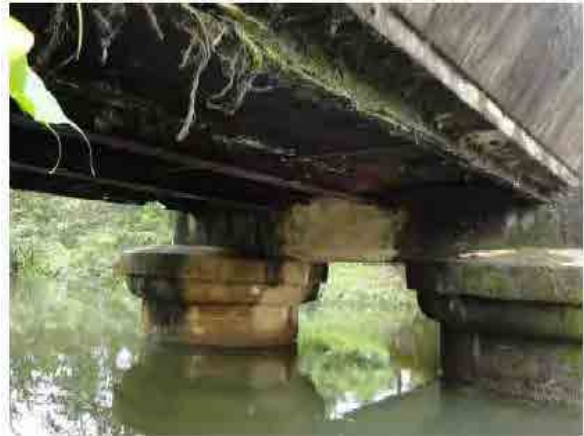
Corrosion and cross sectional deficit of steel main girder Kalutara(B157-23/1)
