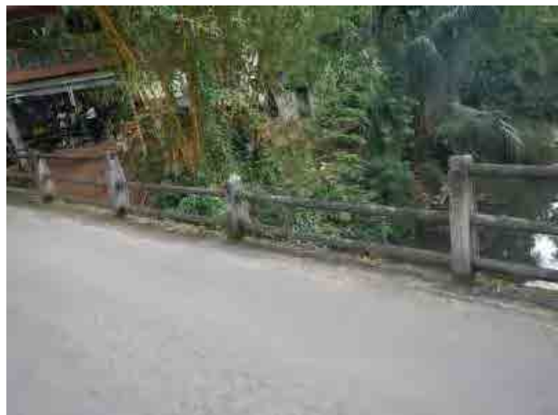
Damage of handrail Matara(B607-10/1)
