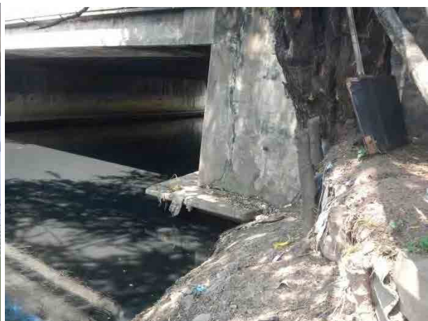
Crack of abutment Colombo(AA001-6/1)
