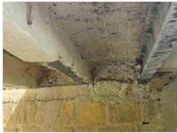
Collapse of lining concrete Kalutara(B224-11/5)
