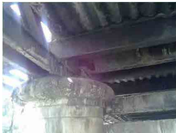
Corrosion of steel main truss and cross beam Kalutara(AA002-20/1)
