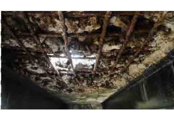
Collapse of floor slab Kalutara(B157-27/8)
