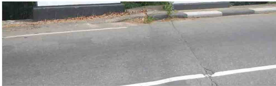
Damage on Existing Expansion Joint
