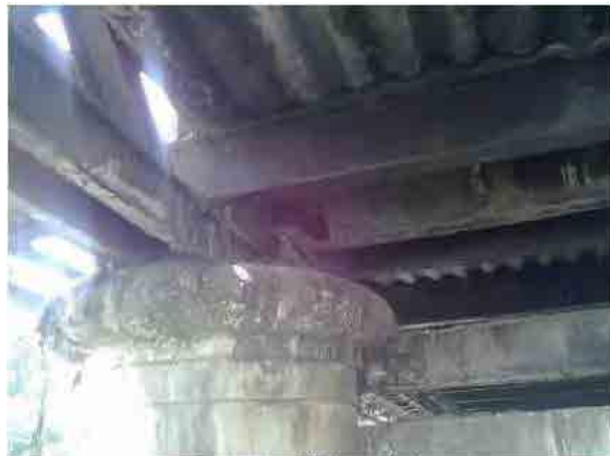
鋼主構・横桁の腐食 Kalutara(AA002-20/1)
