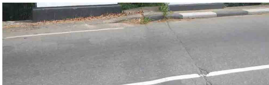
[既存橋梁伸縮部の損傷事例]
