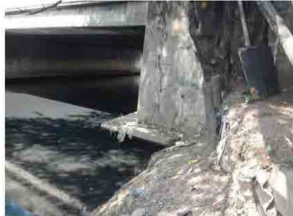
躯体のひび割れ Colombo(AA001-6/1)
