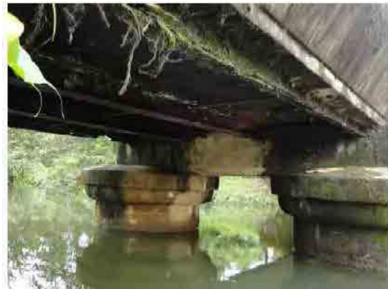
鋼主桁の腐食・断面欠損 Kalutara(B157-23/1)
