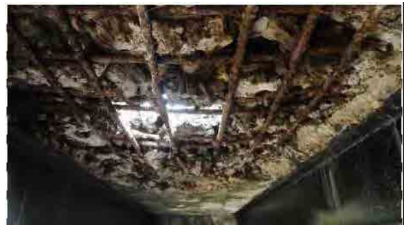
床版の陥没 Kalutara(B157-27/8)
