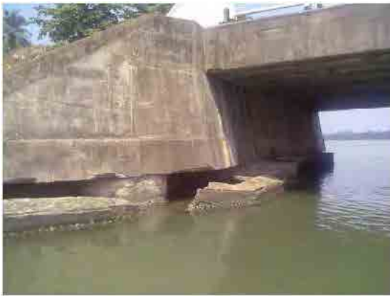
躯体の崩落 Kalutara(AA002-7/1)
