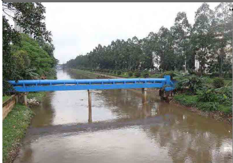
Water supply pipe bridge crossing the river (Banjir Kanal), Banjir Kanal is a river that serves the function of flood adjustment
